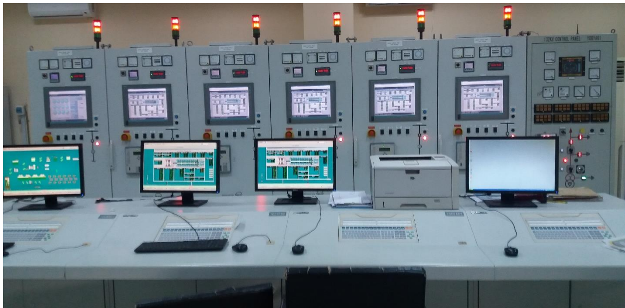
Figure 3.6: Control room of Katakali Power Plant
