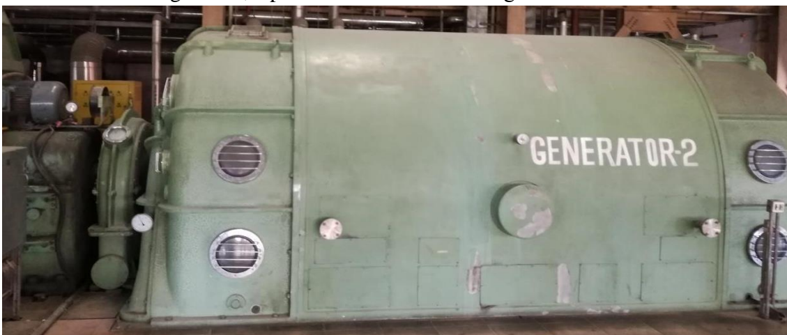
Figure2.3: Generator of Barapukuria 125 MW unit
