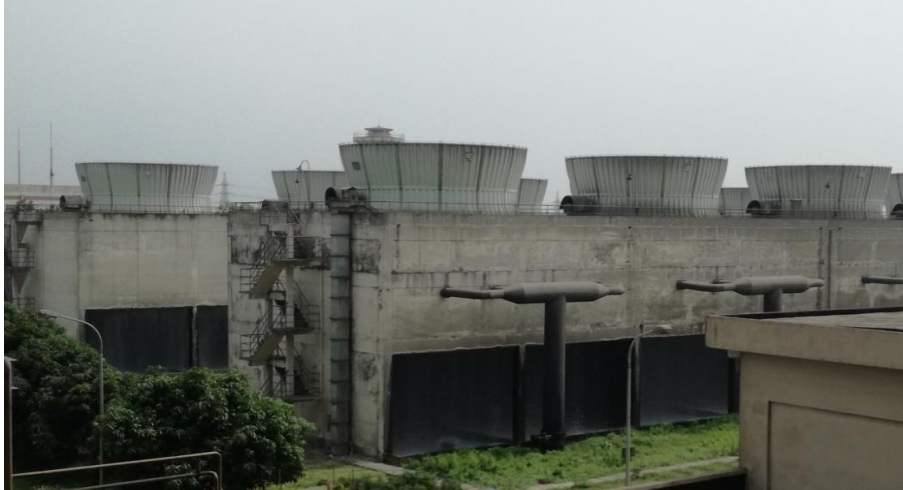
Figure2.5: Water cooling towers of Barapukuria 125 MW unit
