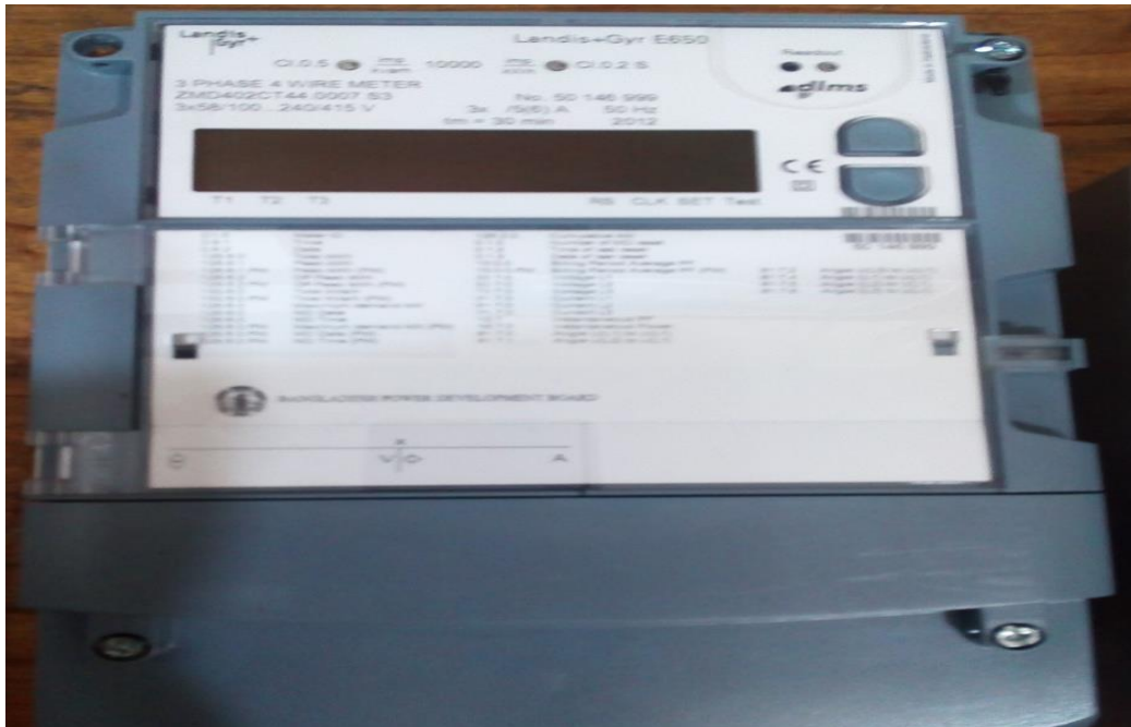
Figure 6.2: High Tension Meter
