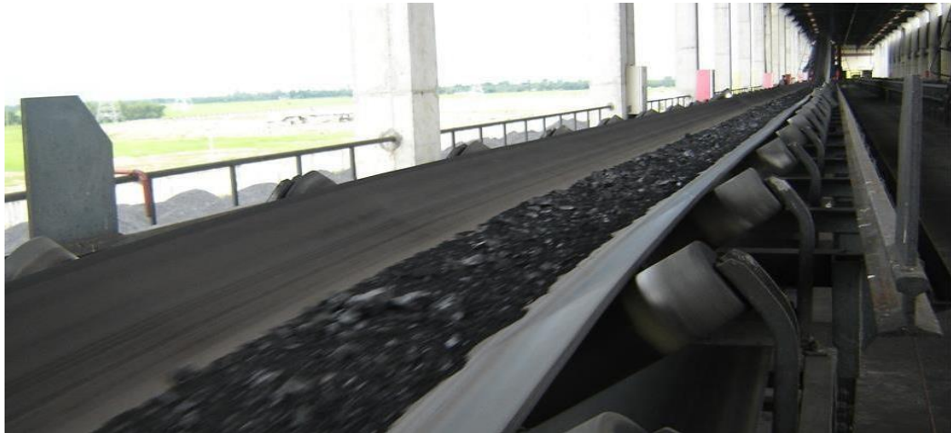
Figure 2.1: Conveyer belts for coal transport at Barapukuria
