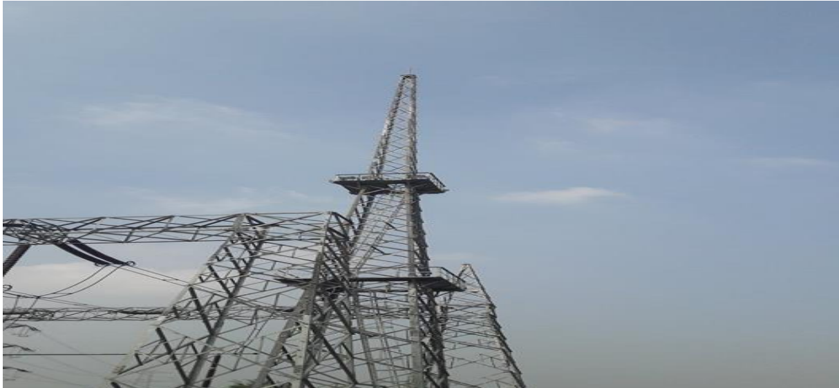
Figure 5.3: Lightning Arrester of (HVDC) Grid Substation
