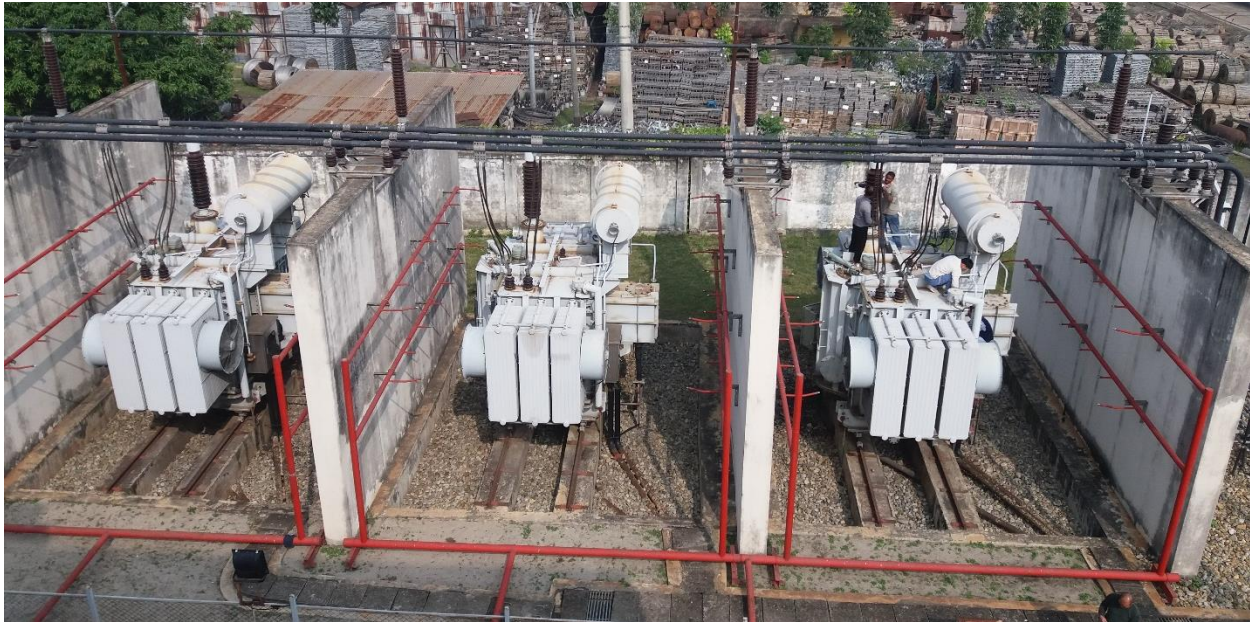
Figure 3.4: 11/132KV transformer at Katakali Power Plant
