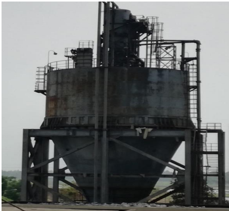
Figure 2.6: Ash collector at Barapukuria Power Plant
