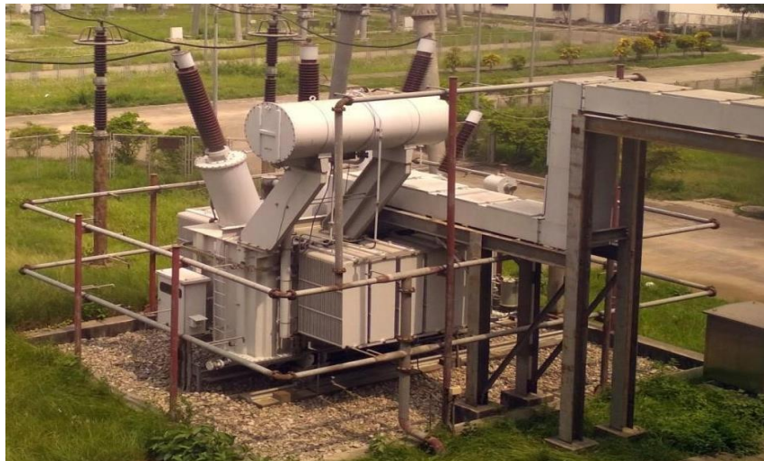
Figure 2.4 Power transformer of Barapukuria
