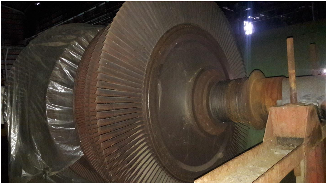
Figure 4.3: Turbine blades for 60 MW unit at Khulna power plant [2]
