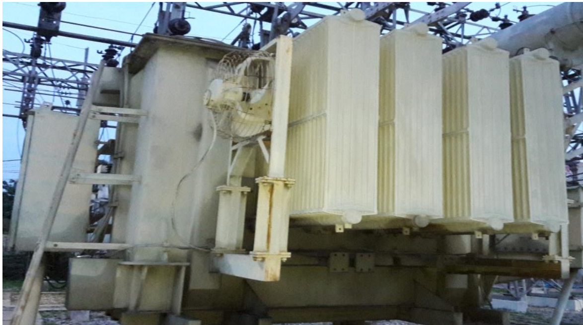
Figure 5.5: 33/11KV power transformer at Horogram substation [2]
