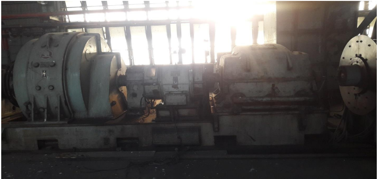
Figure 4.2: Side view of 60 MW generator at Khulna power plant [2]
