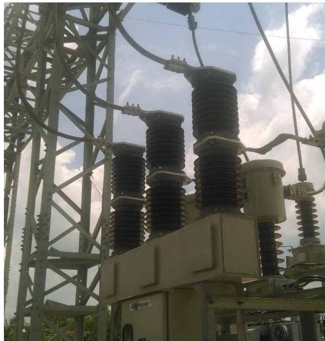
Figure 5.7: Vacuum circuit breaker at Horogram Substation [2]
