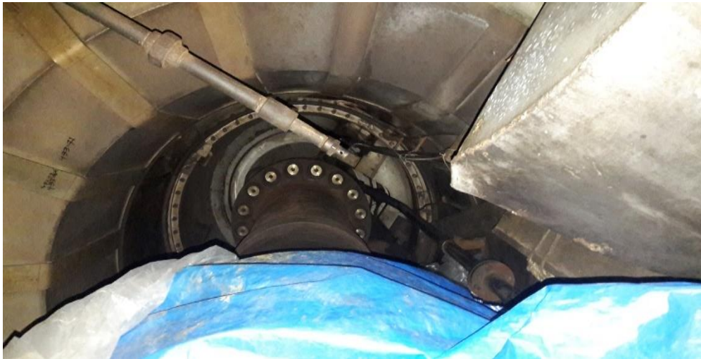
Figure 3.3: The coupling part of gas turbine with generator at Baghabari power plant [2]
