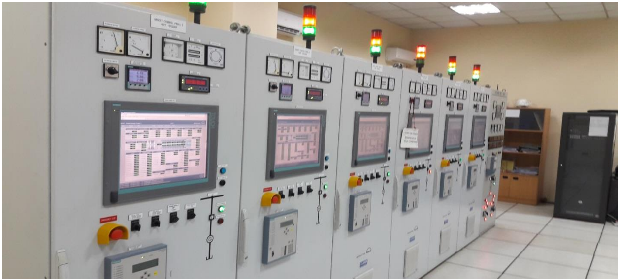
Figure 2.6: Monitoring section of control room (Katakali power plant) [2]
