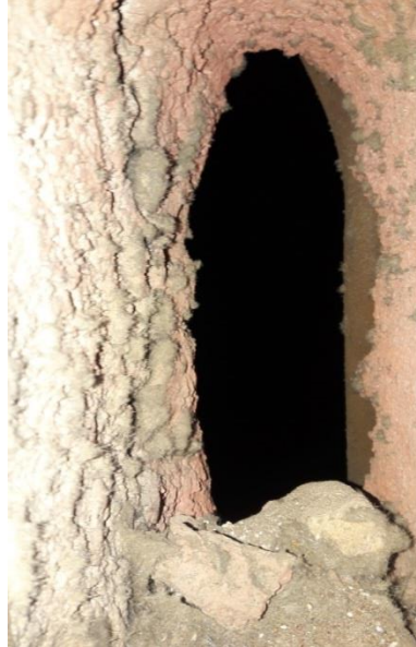
Figure 4.4: The opening gate of furnace at Khulna power plant [2]
