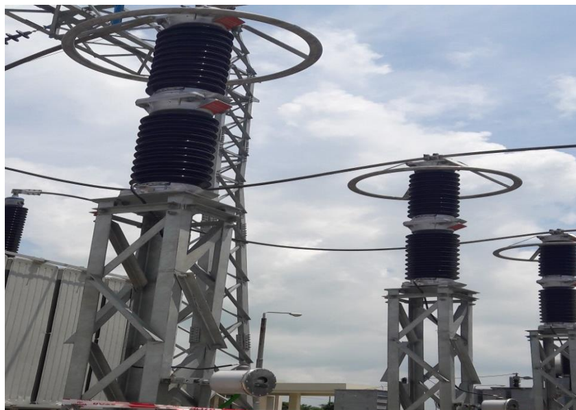
Figure 5.9: Lightning arrester at Amnura grid project [2]
