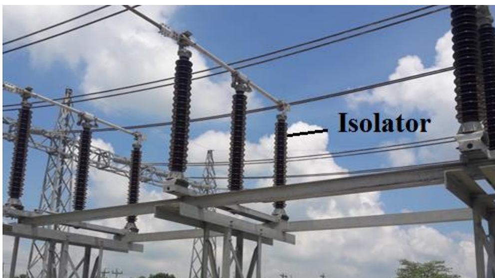
Figure 5.3: Isolator at Amnura grid project [2]
