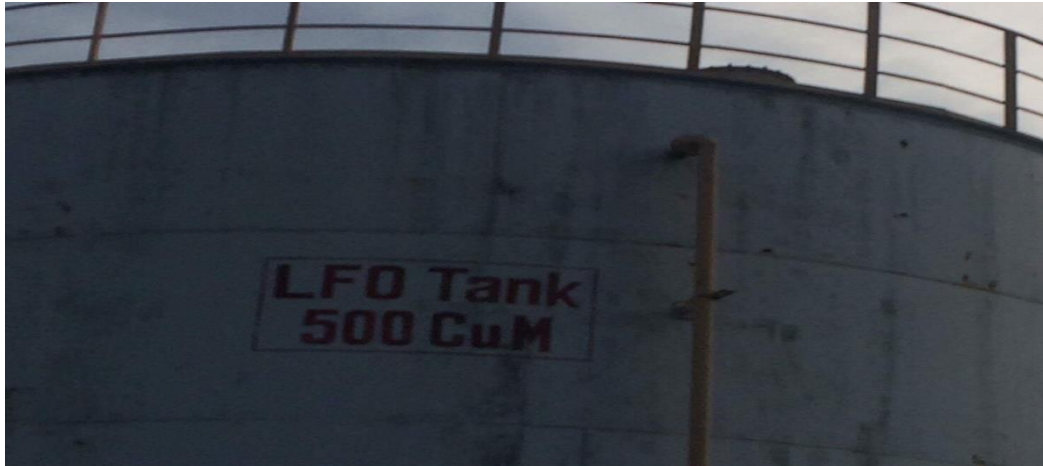
Figure 2.3: Storage tank for LFO at Katakali power plant [2]
