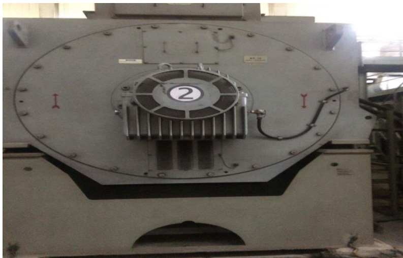
Figure 2.4: Front view of the diesel Engine at Katakali power plant [2]
