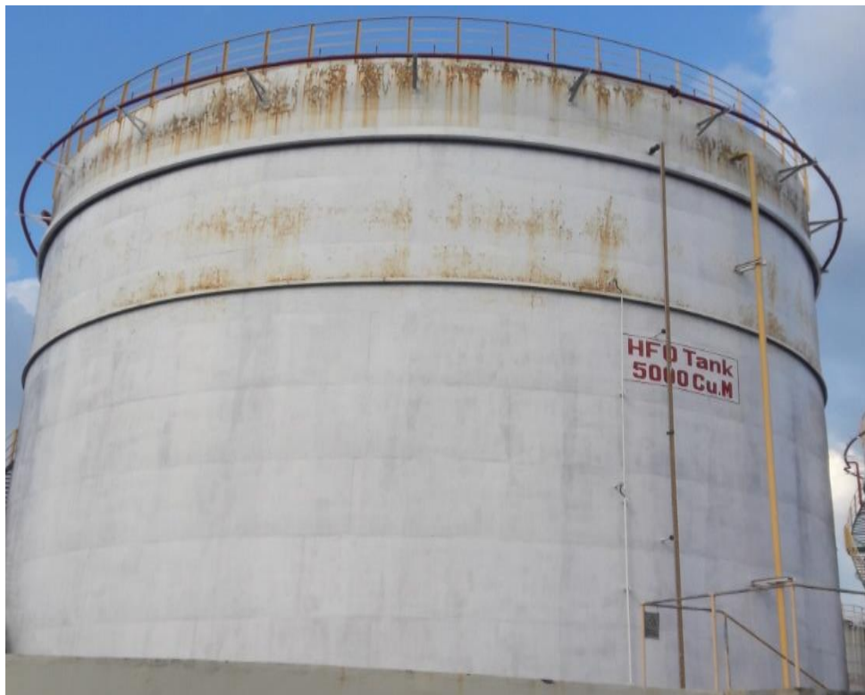
Figure 2.2: Storage tank for HFO at Katakali power plant [2]
