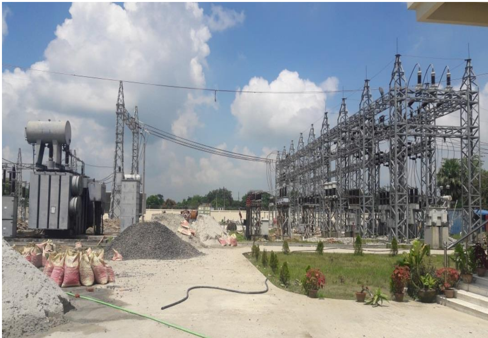
Figure 5.1: Double bus bar at Amnura grid project [2]
