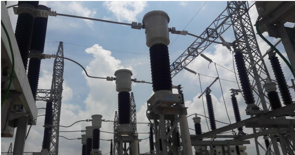
Figure 5.6: Current transformer at Amnura grid project [2]
