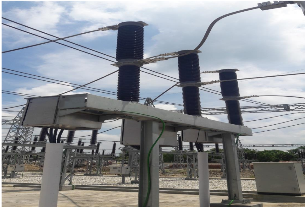
Figure 5.8: SF 6 circuit breaker at Amnura grid project [2]
