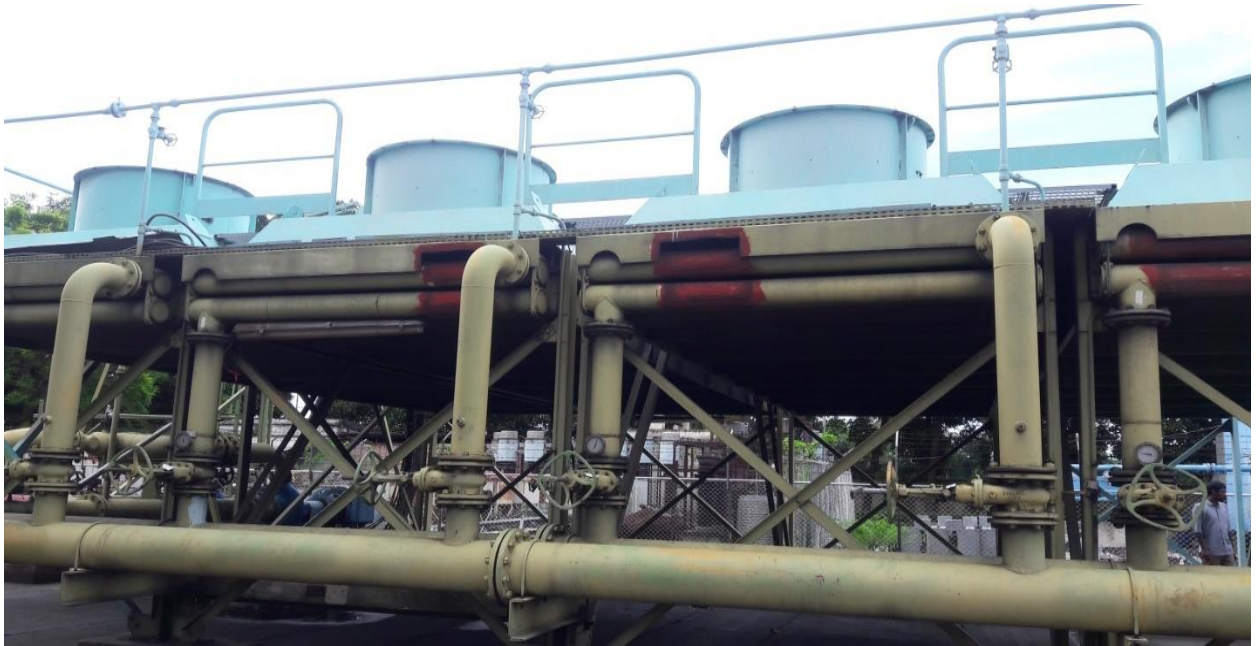
Figure 3.4: The front view of lube oil system at Baghabari power plant [2]
