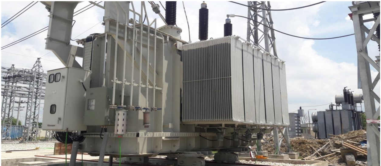
Figure 5.4: 132/33KV power transformer at Amnura grid project [2]
