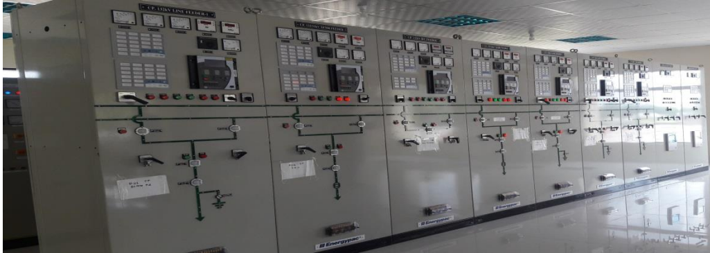
Figure 5.10: The front view of relays in control room at Amnura grid project. [2]
