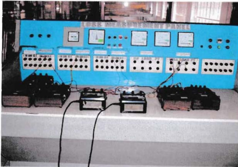
Figure -: A screenshot of No load test Equipment panel
