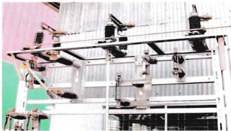
Figure -: A snapshot of switches displayed at Energypac
