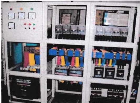
Figure -: A screenshot of LT switchgear manufactured at Energypac
