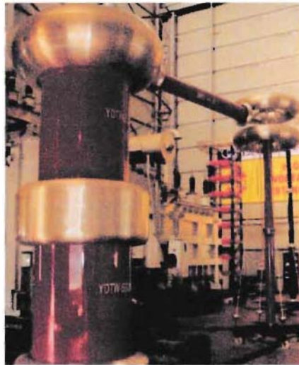
Figure -: High voltage test components
