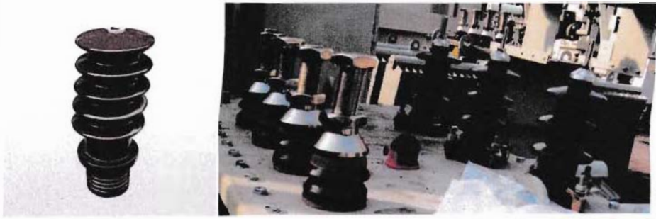
Figure -: Bushing of a transformer
