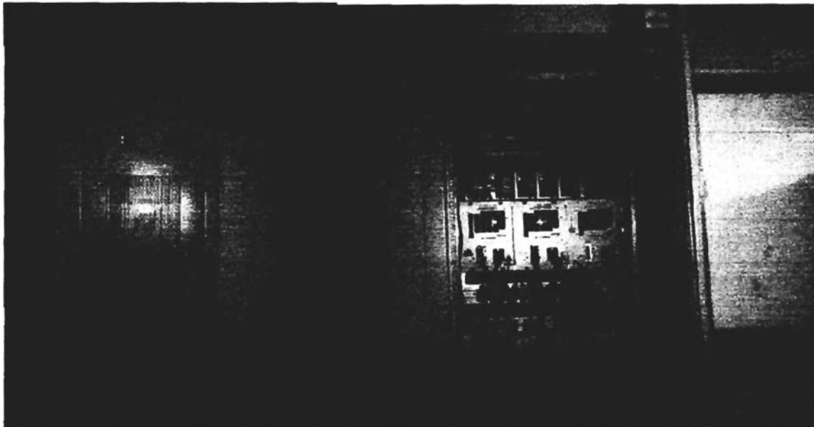
Figure 10: BSMC Rectifier system with 50 amp modules.
