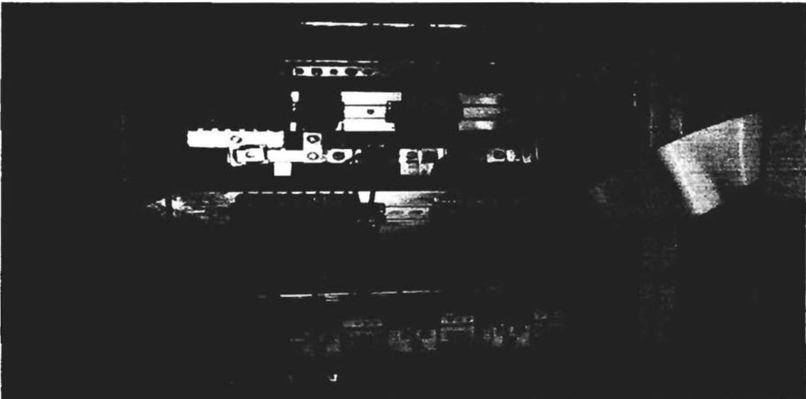
Figure 15: ASCOM rectifier with 2000 W modules (2 LVD System)
