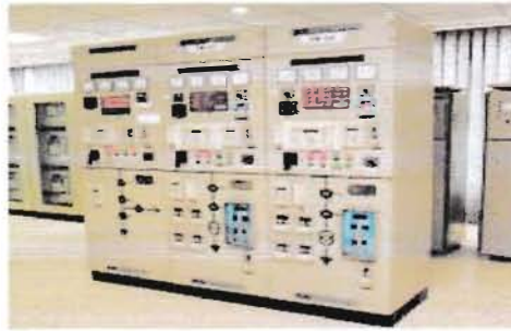
Figure 29: Control Relay Panel (www.energypac.com)
