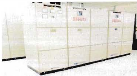
Figure 28: PFI plant ( www.energypac.com )
