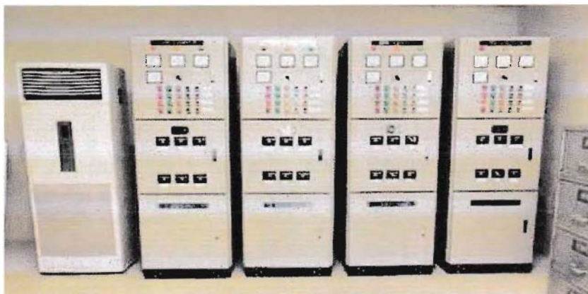
Figure 16: LT switchgear panel
