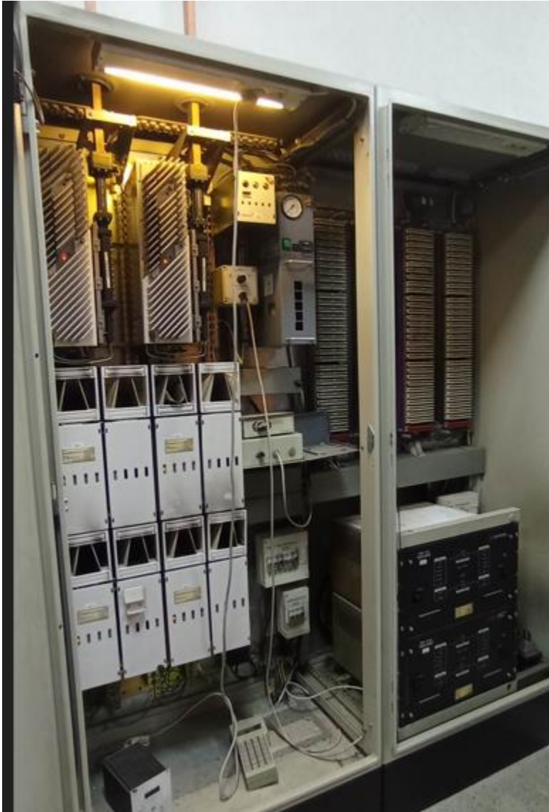
Figure-4: SCADA Communication Equipment
