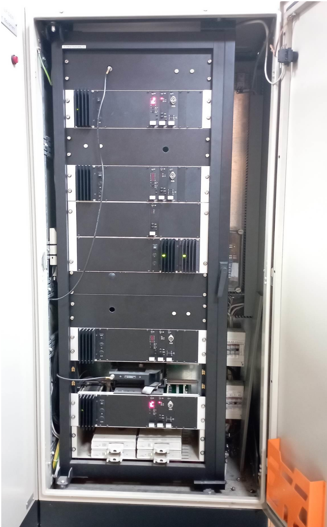
Figure-3 : SCADA Communication Equipment
