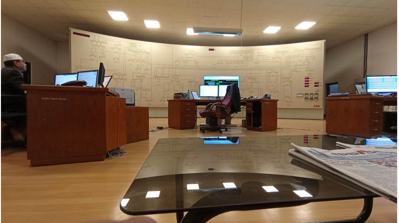
Figure-1 : SCADA panel of DPDC
