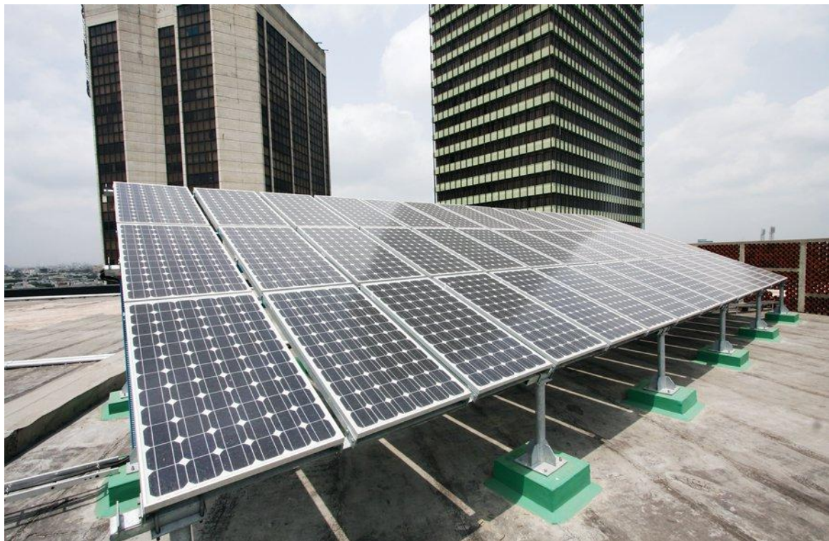
Figure 4.1: Solar Photovoltaic (PV) in DPDC Held Area
