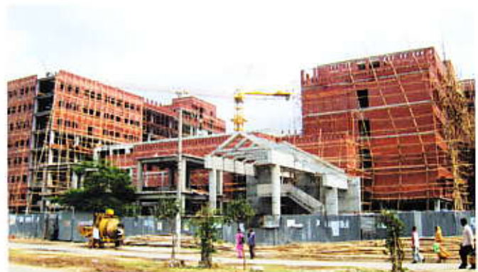
The construction work of the permanent campus of East West University at Aftabnagar is going on in full speed.
