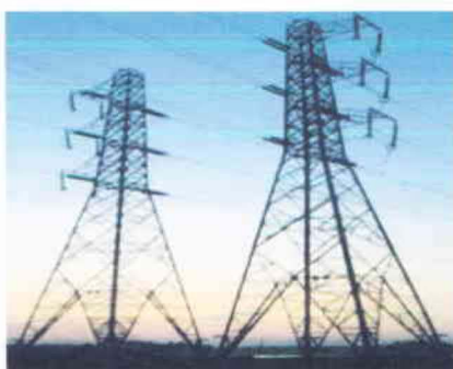
Figure 3.19: High Voltage Tower
