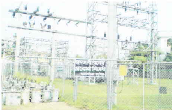
Figure 3.21: Overall View of the Distribution Substation
