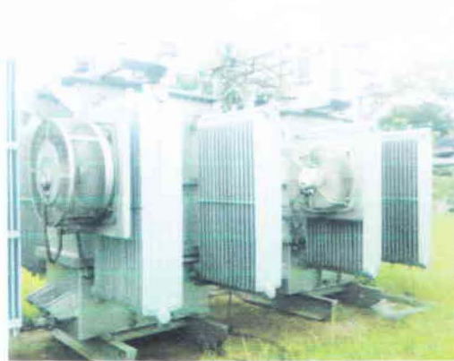
Figure 4.5: A transformer with cooling fan
