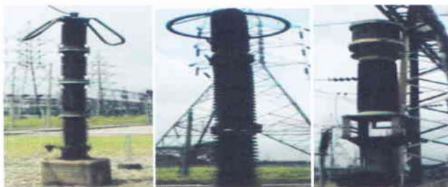
Figure 3.12 Picture of Lightning arrestor
