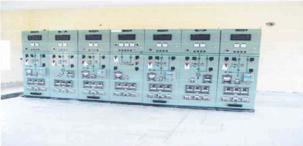
Figure 4.16 : Programmable Logic Control Unit
