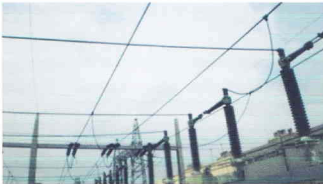
Figure 3.8 An Isolator which is used for Maintenance Purpose
