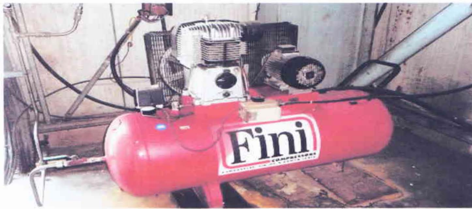
Figure 3.3: The Compressor of GT-1
