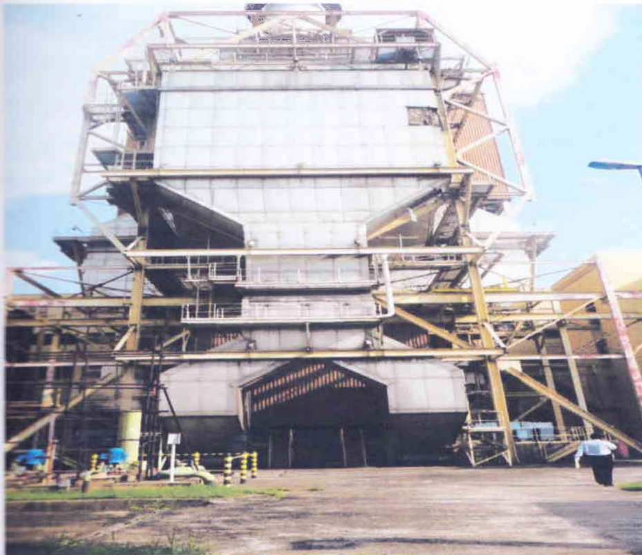
Figure 2.1: Water Tube Steam Boiler of APSCCL
