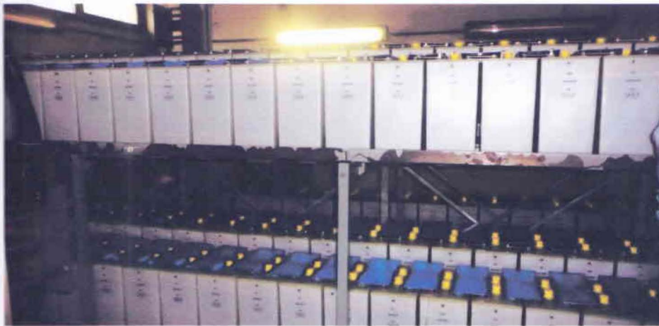
Figure 2.8: Batteries of Ashuganj Power Plant for back-up System
