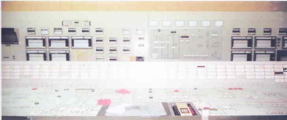
Figure 2.10: Control Room of unit 2 & 5
