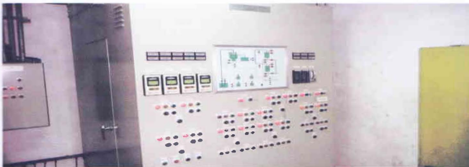
Figure 2.4: Control room of filter house
