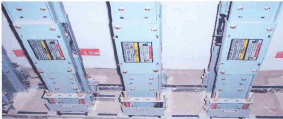
Figure 2.14: Bus bars used in APSCCL
