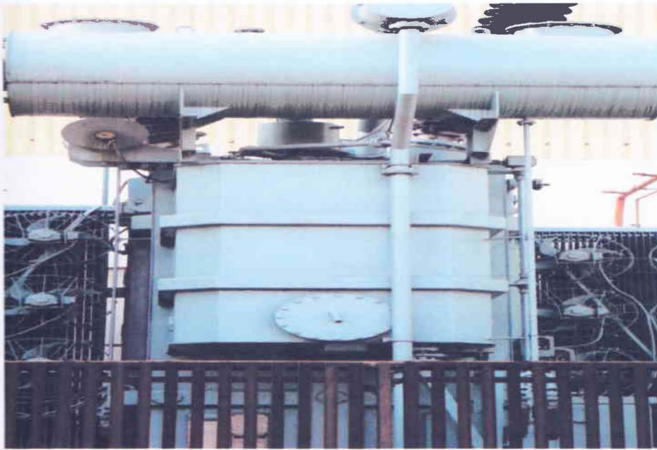
Figure 2.9: External Cooling System of transformer
