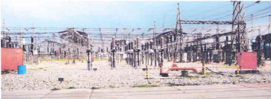
Figure4.1: Substation of APSCCL
