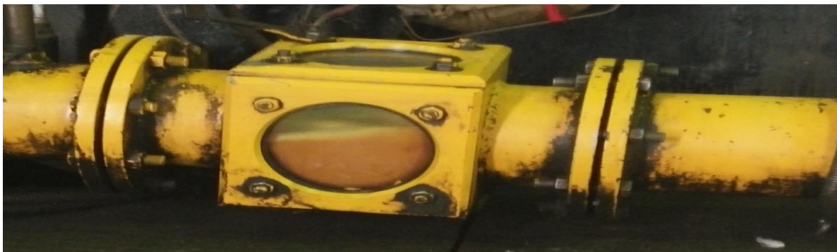
Figure 4.16: Lubrication oil supply.
