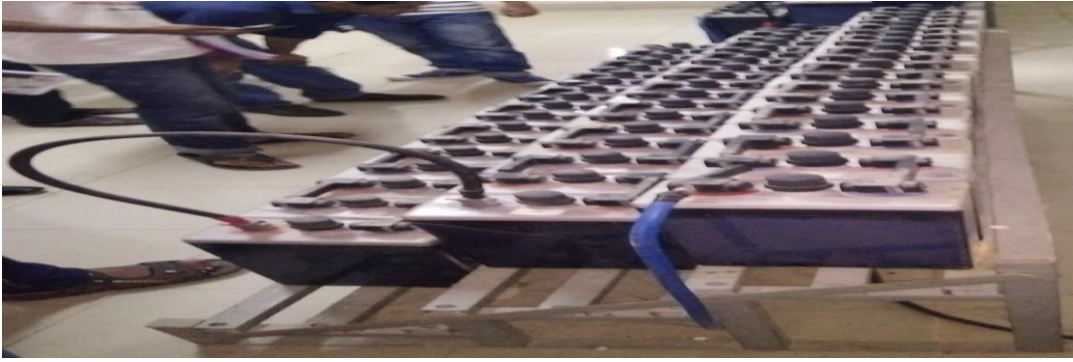
Figure 5.7: Battery bank for initial excitation.
