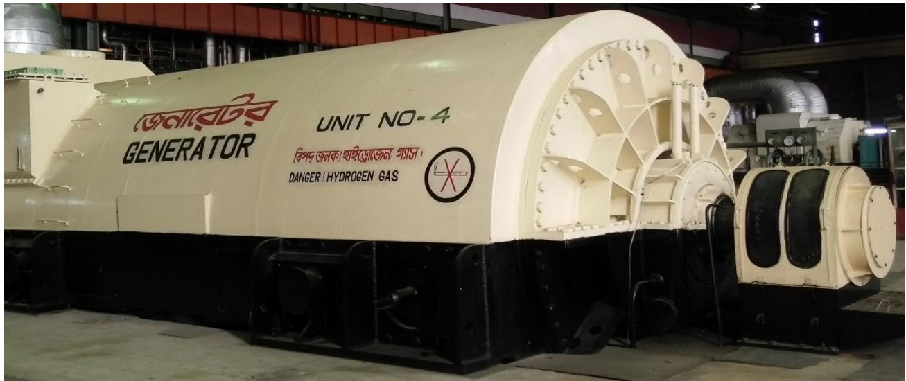
Figure 5.1: Generator at GPS (Unit-4).
