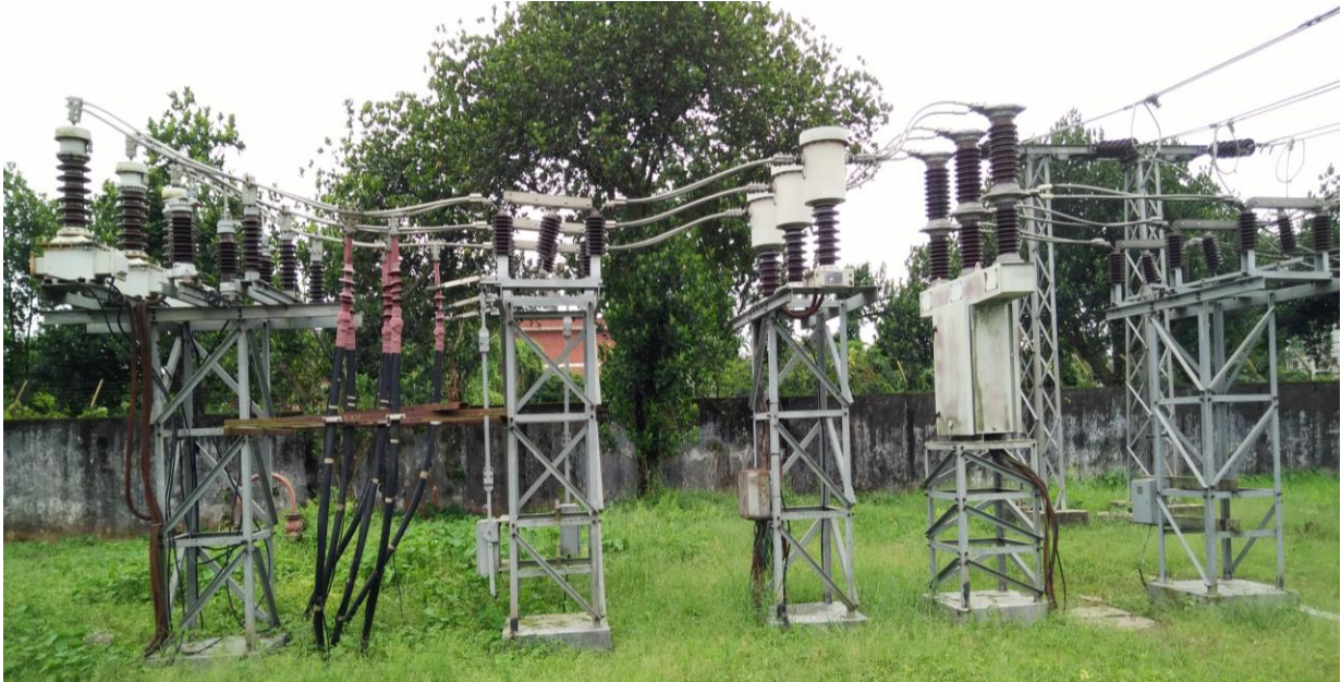
Figure 6.15: Incoming feeder bay at GPS.
