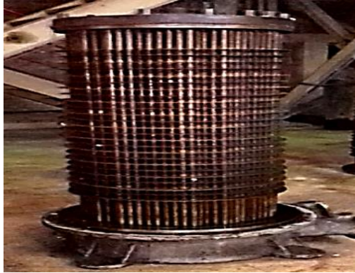
Figure 3.2: Economizer of unit-6 at GPS.
