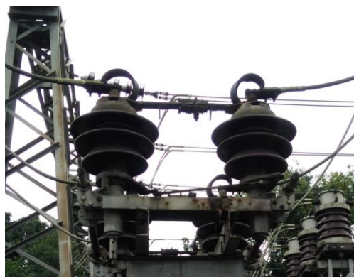
Figure 6.19: Isolator at GPS.
