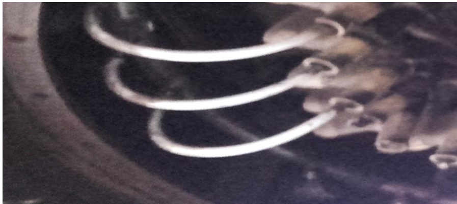
Figure 5.6: Stator water pipes.
