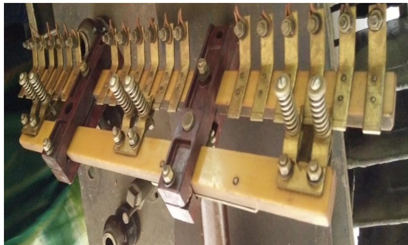
Figure 6.10 : Transformer Tap Changer.
