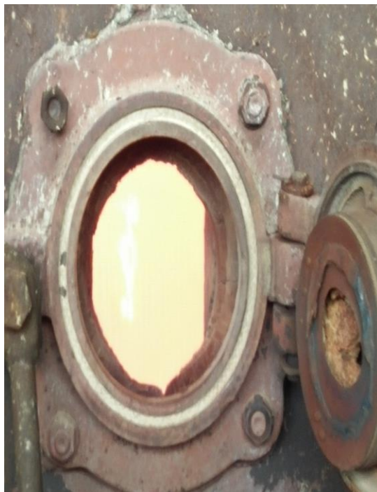
Figure 3.1: Furnace of unit-3 at GPS.
