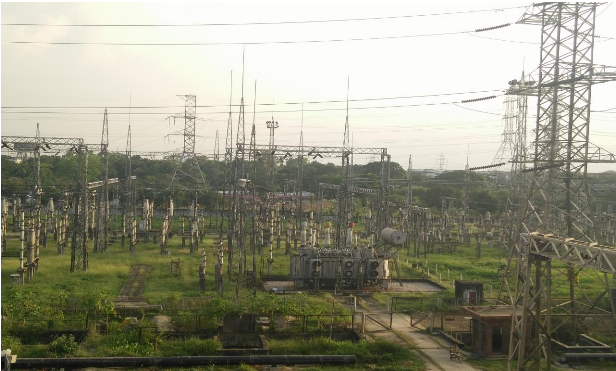
Figure 6.1: Sub-station of GPS.
