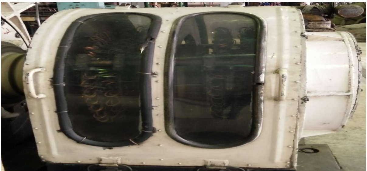
Figure 5.5: Carbon brush and slip ring chamber (Unit-4).
