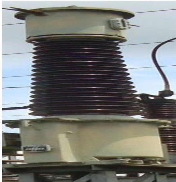
Figure 6.7 : Potential transformer (PT).
