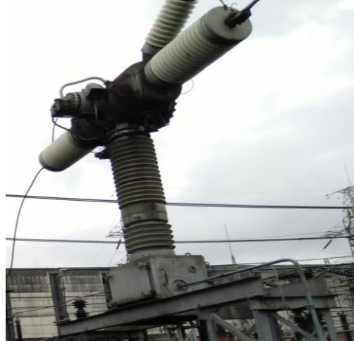
Figure 6.16: Air blast circuit breaker (ABCB).
