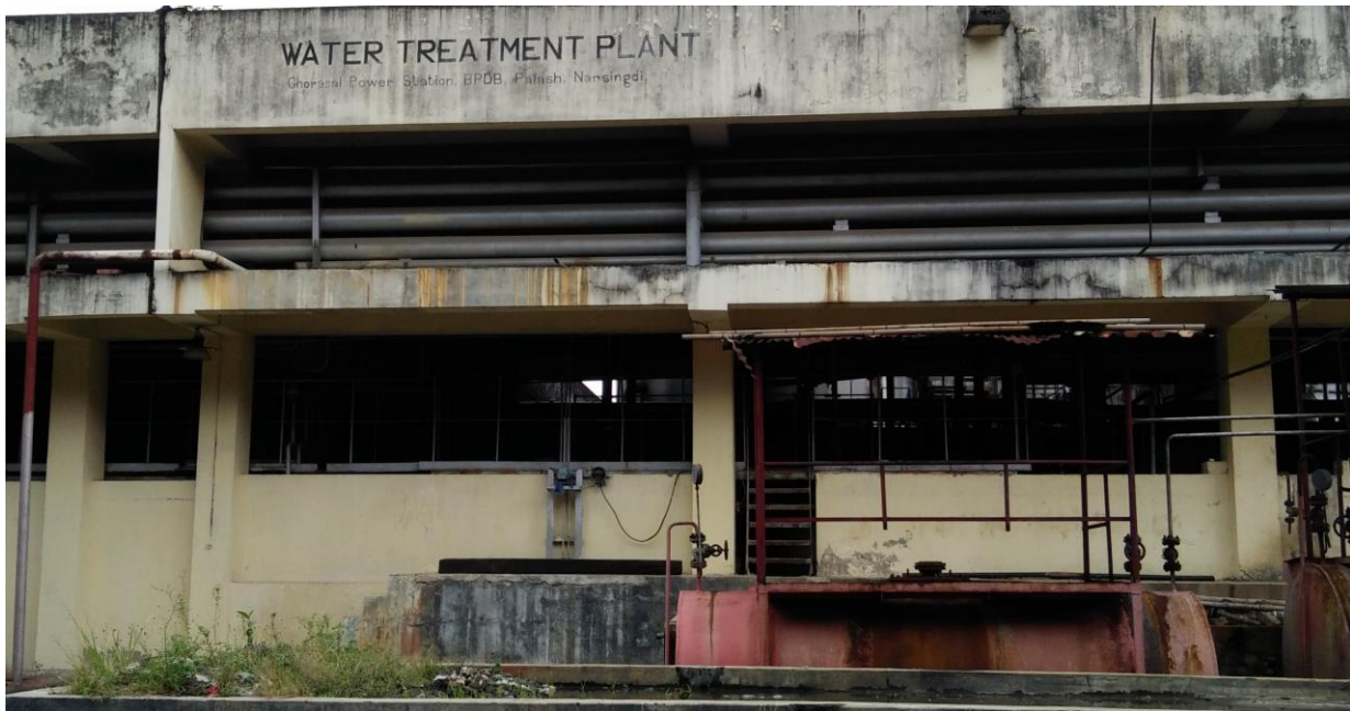
Figure 2.1: Water treatment plant of GPS.
