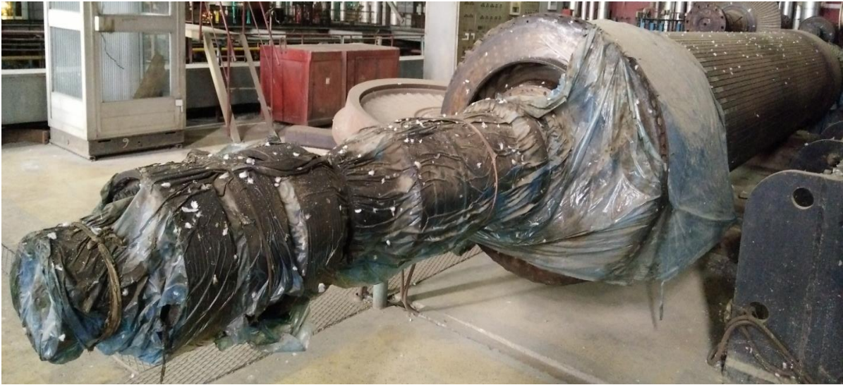
Figure 5.4: Rotor of unit-6 at GPS.
