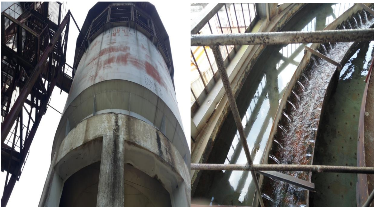
Figure 2.2: Clarifier of GPS.
