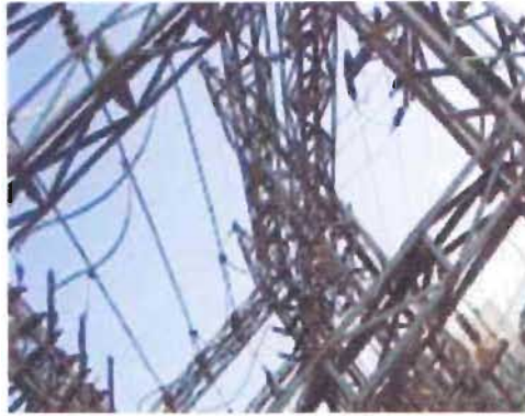
Figure 3.2: Bus-Bar of Substation(double bus bar arrangement)
