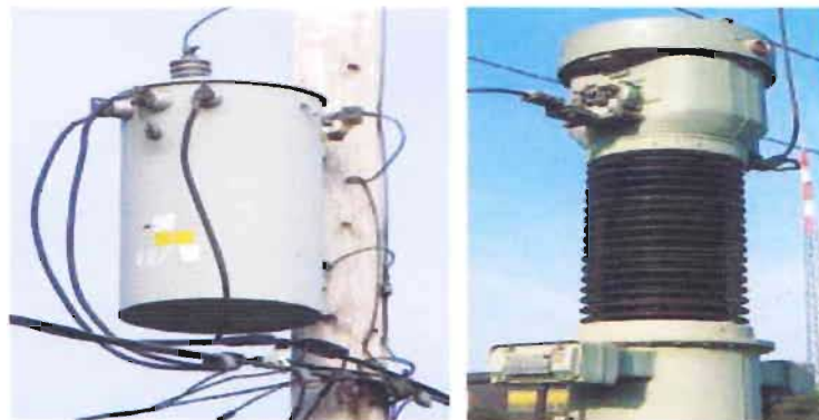
Figure2.3: Current Transformer rating 150:5(Pole mounted and 11KV)
