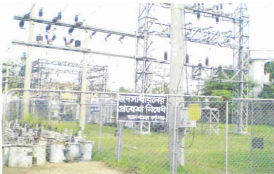
Figure 4.2: Overall View of the Distribution Substation
