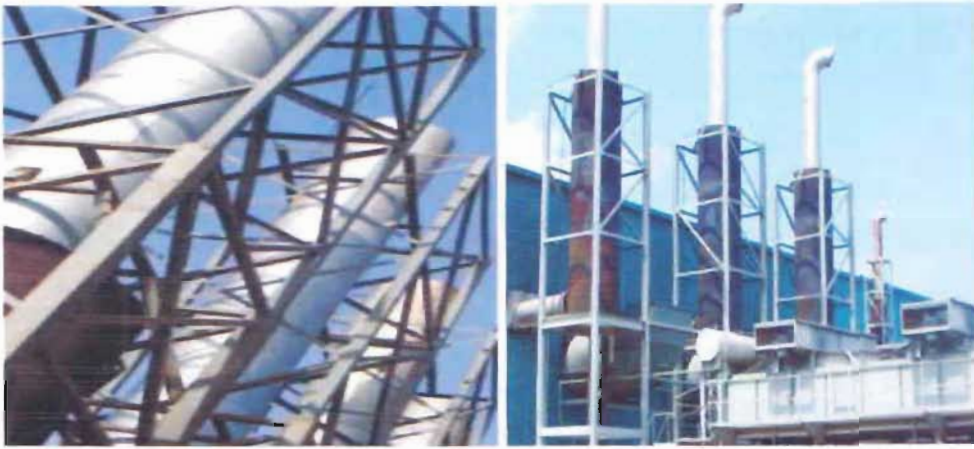
Figure 2.7: Radiator(with 14 fans) exhaust at UPGD
