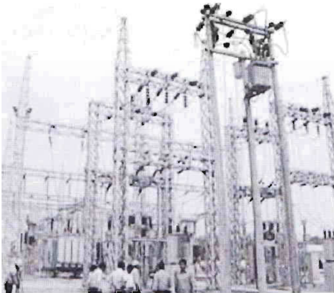
Figure 2.1 : Grid and substation operation
