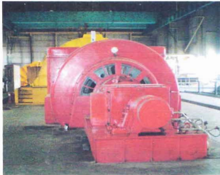
Figure 2.1: Picture of AC generator (64MW) of unit 2
