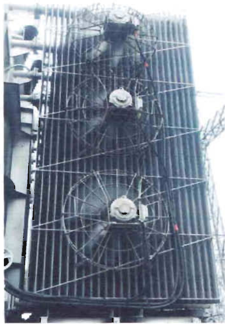
Figure 4.3: Air Cooling of generator transformer.
