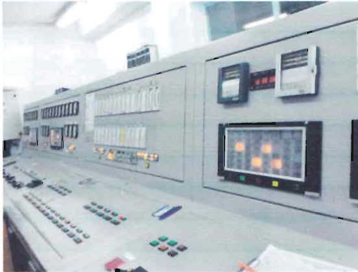
Figure 7.11: Control unit of combine cycle plant.
