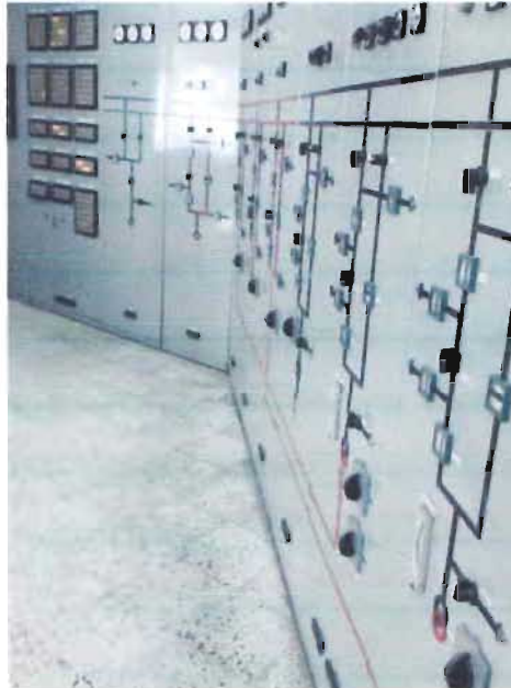
Figure 7.13: Control unit of sub-station.
