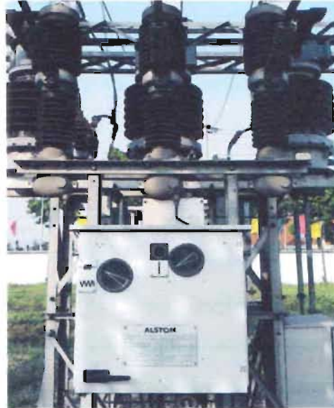
Figure 5.6: Picture of oil circuit breaker.
