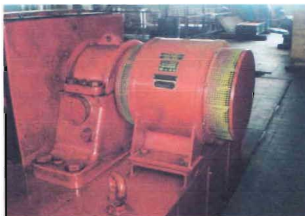
Figure 2.3: Outlook picture of AC excitation system of 64MW (Unit 2)
