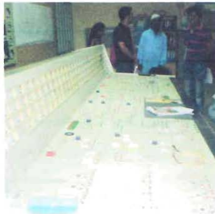
Figure 7.3: Operation unit of control unit 3
