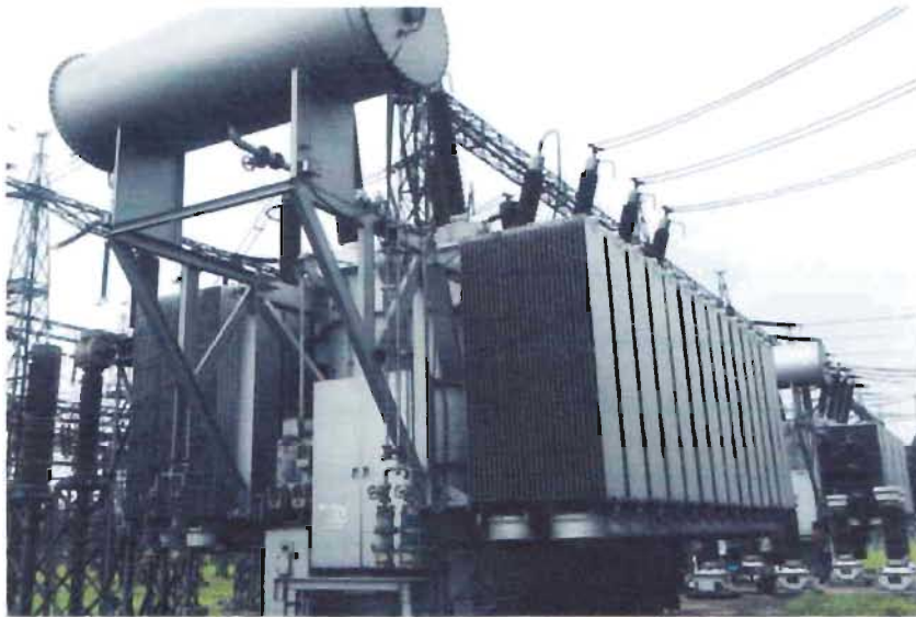
Figure 5.1: Picture of a Power Transformer of 132 KV line
