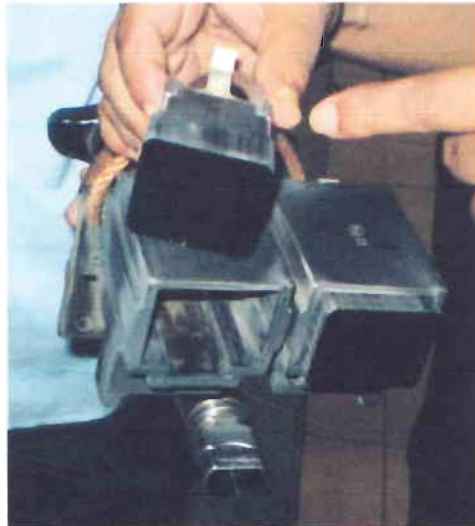
Figure 2.2: Brush of DC exciter of unit 3.
