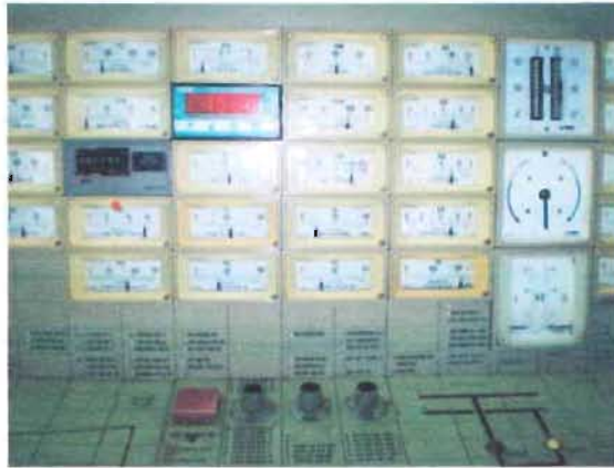
Figure 7.2: Various Parameters monitoring room of control unit 3
