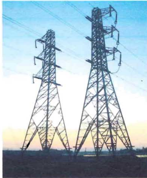
Figure 5.9: Distribution line (11KV) of APSCL
