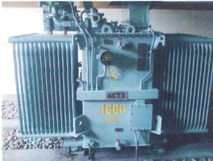
Figure 3.11: Picture of Unit Transformer.
