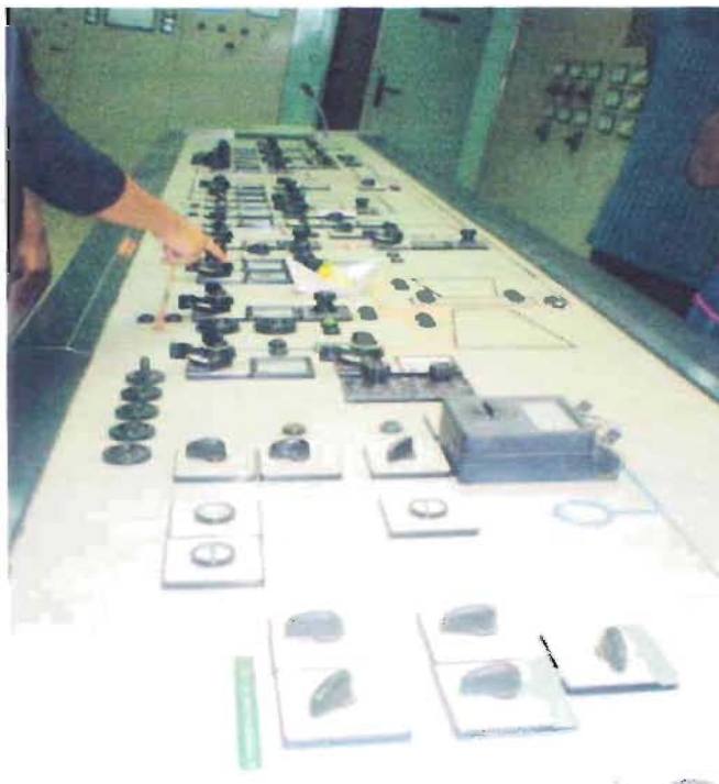
Figure 7.4: Operation unit of control unit 1 & 2
