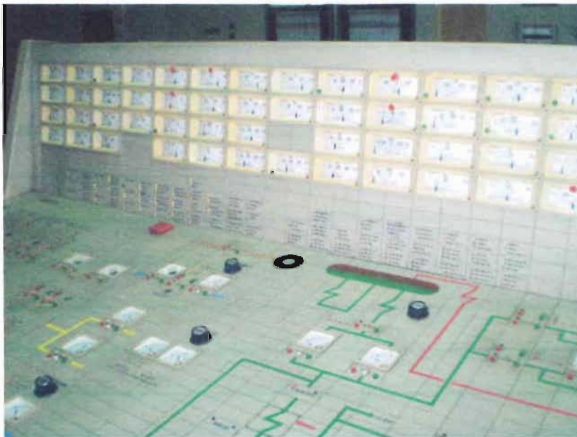
Figure 7.8: Control unit of 3 and 4
