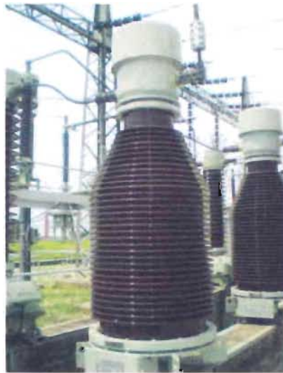
Figure 5.2: Picture of a Current Transformer of 132 KV line
