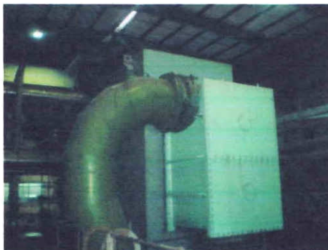
Figure 2.15: Condenser used in steam turbine section of combined cycle power plant converting heat energy of steam into mechanical energy in the prime mover. Secondly, the condensed steam can be used as feed water to the boiler.
