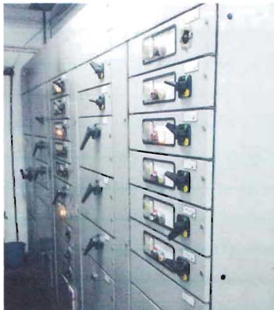
Figure 7.12: Switchgear unit of combine cycle plant.
