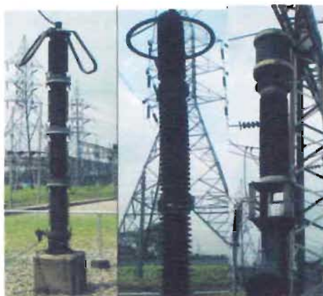
Figure 5.8: Picture of Lightning arrester.
