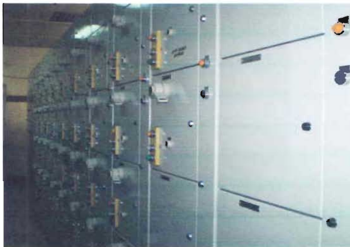
Figure 7.1: Switchgear room of control unit 3
