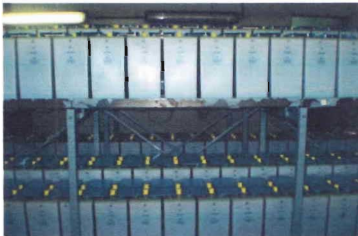
Figure 5.11: Battery arrangement of back up system
