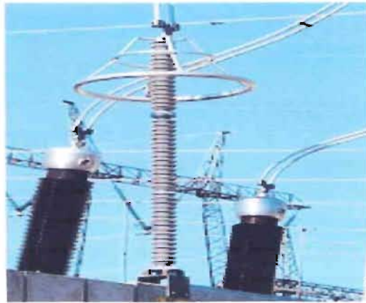
Figure 4.8: Lightning Arrester in the substation; which protect equipments from lightning
