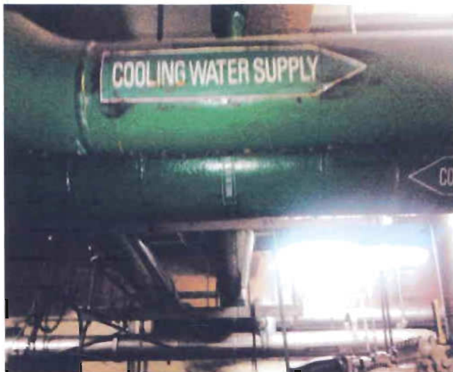
Figure 3.13: Cooling water supply pipe in APSCL
