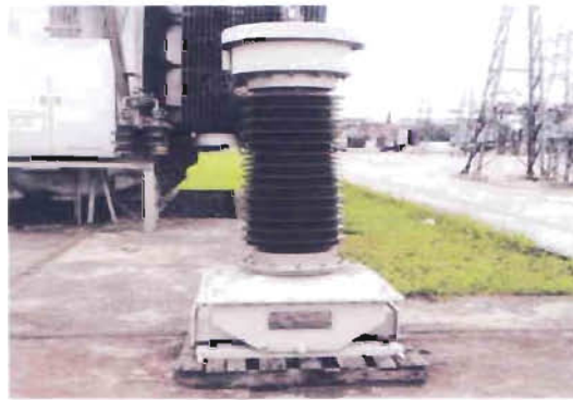
Figure 4.3: Current Transformer used in APSCCL's substation
