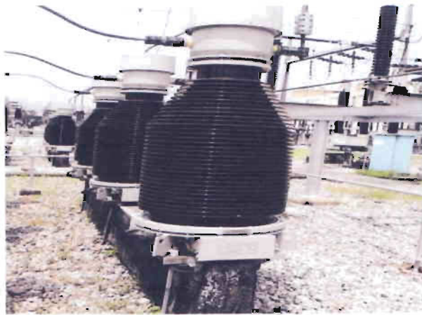
Figure 4.4: 132 kV single phase outdoor types Potential Transformer used in APSCL substation
