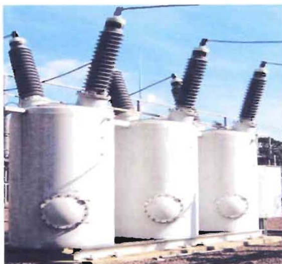
Figure 4.5: 132 KV rated voltage Minimum oil Circuit Breaker used in APSCS substation
