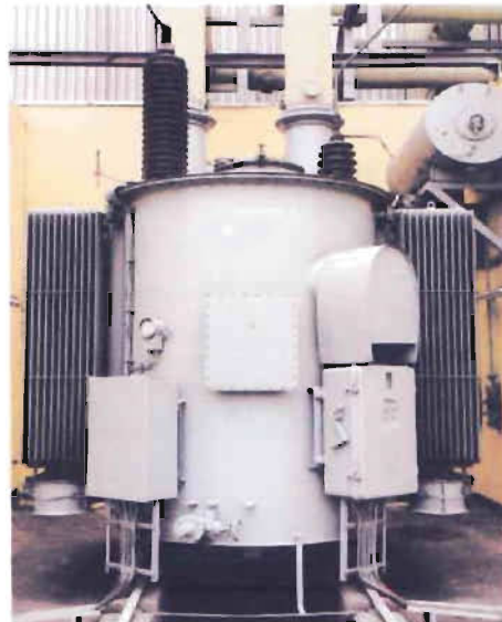
Figure-4.2: An on-load tap-changing transformer, changed voltage level from 15.6 kv to 132 kv
