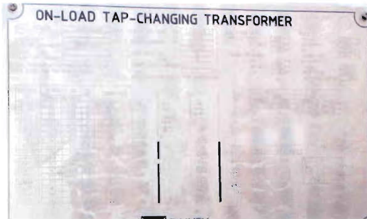
Figure-4.1: Name plate data of an on-load tap-changing transformer used in APSCL
