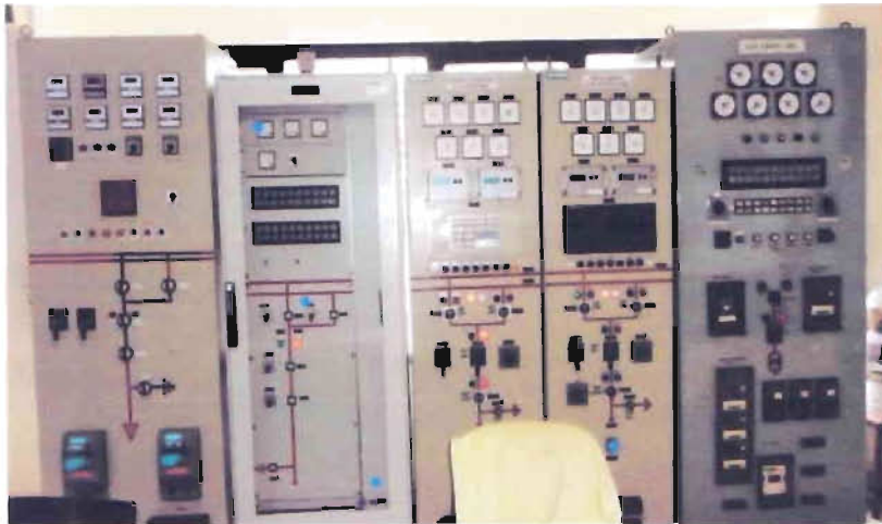
Figure-4.10: Control room of substation in APSCL
