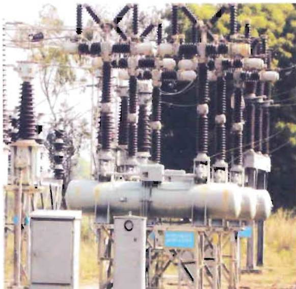
Figure 4.7: Air blast Circuit Breaker used in APSCL's substation for protection [13]
