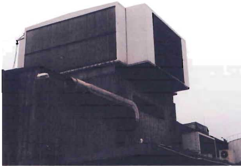
Figure 3.14: Air Inlet system in gas turbine in APSCL
