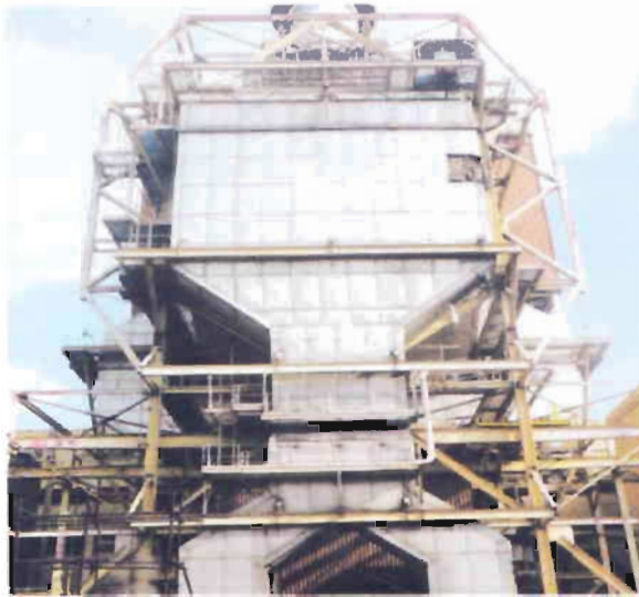
Figure 2.2: Boiler (unit-3 and its capacity is 150MW)
