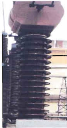
Figure 4.9: Wave Trap in the substation; which is used for communication in APSCL
