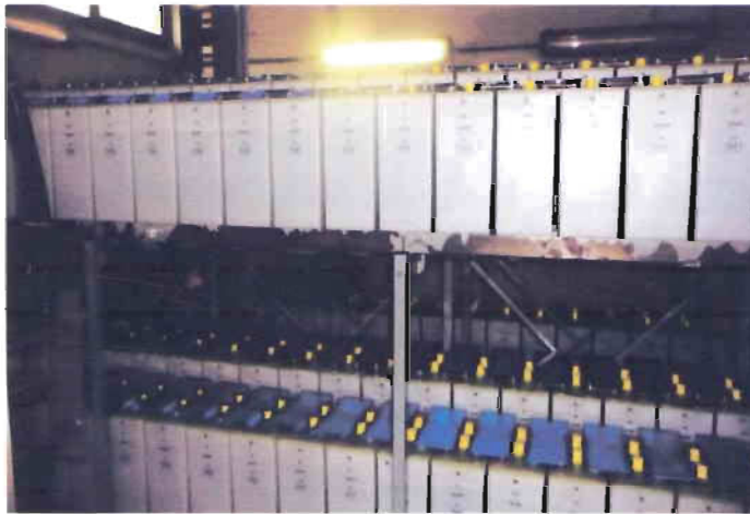
Figure 2.14: series connected battery (No of batteries: 184, Voltage level of each battery: 1.2v, Total voltage: 220v)
