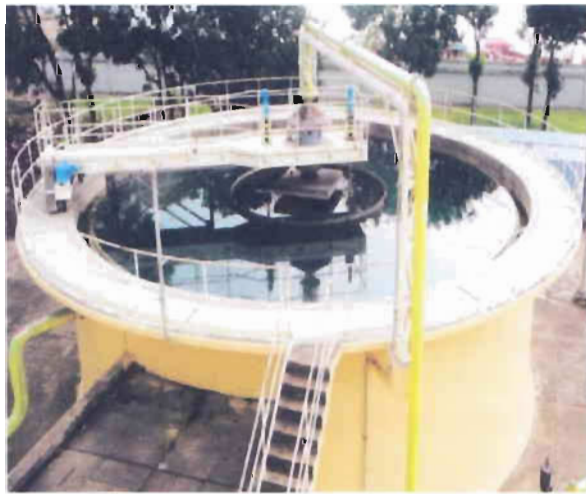
Figure 2.3: 2 stages water purifying basin (is used to reduce the dust from the river water)
