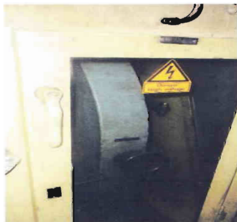
Figure 2.9: Jacking oil pump (is used to cool the shaft and eliminate rotor distortion)
