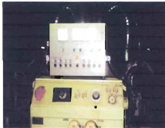
Figure 2.7: Generator (Brown Boveri Company) of APSCL
