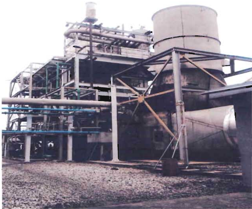
Figure 3.11: Water cooling system of the generator
