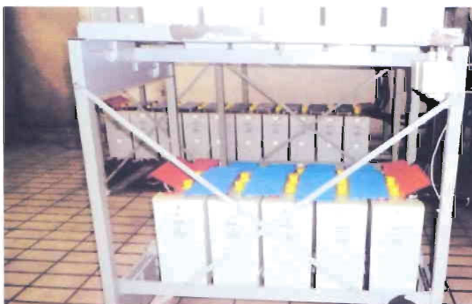
Figure 2.15: parallel connected battery (+24v to -24v, Used to increase the capacity of the series connected battery)
