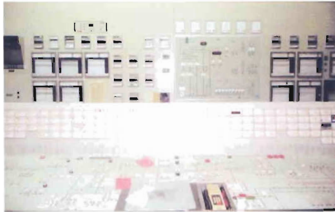
Figure 2.16: Control room of steam power plant of unit-3, 4
