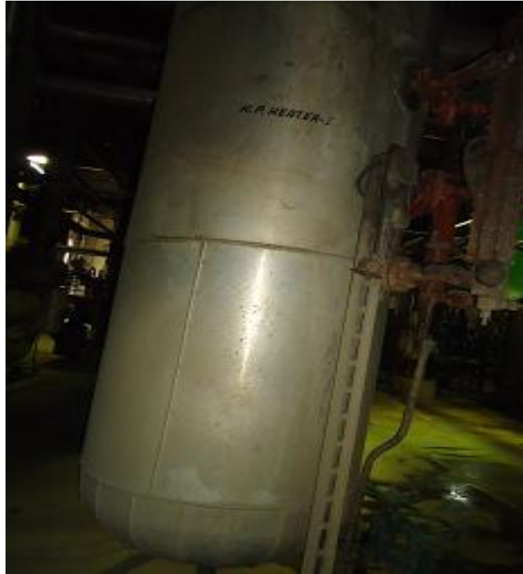
Figure 2.15: High pressure heater.
