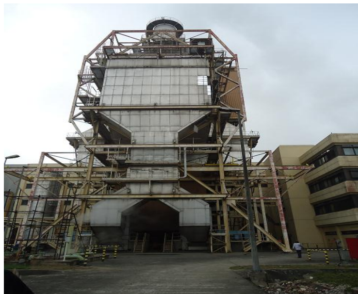
Figure 2.4: Boiler section of steam turbine unit 4.
