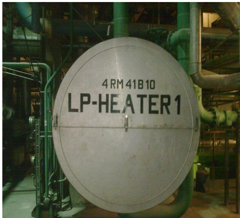
Figure 2.14: Low pressure heater.
