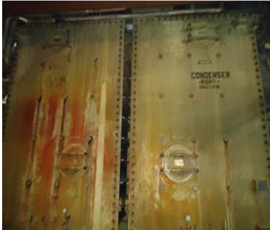
Figure 2.12: Left condenser and right condenser.
