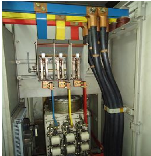
Figure 3.4: A rectifier unit.
