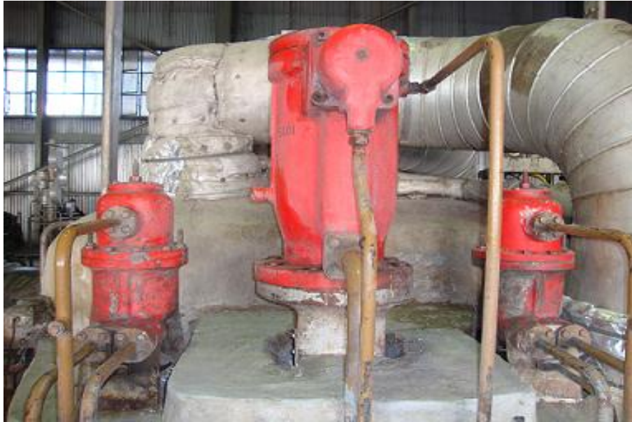
Figure 2.11: Main stop valve (middle) and regulating valves (left and right).
