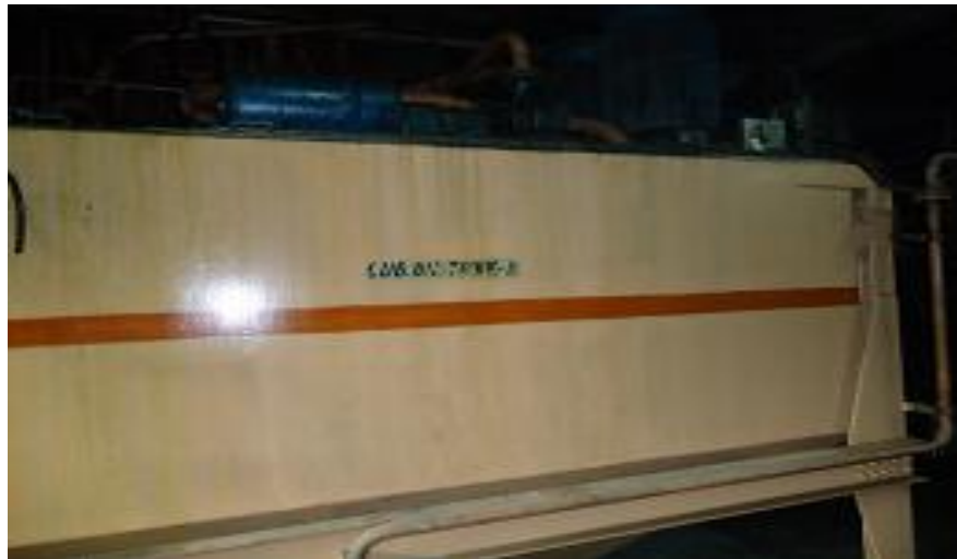
Figure 2.16: Lube oil tank.
