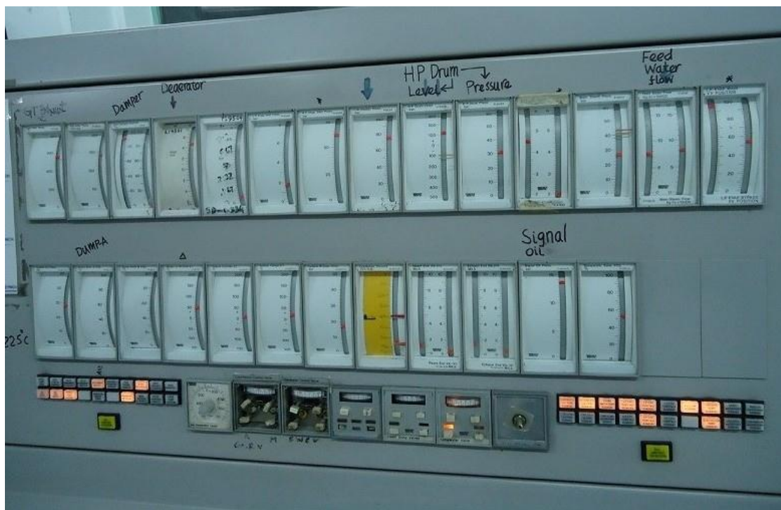
Figure 6.1: Panel board of combined cycle power.
