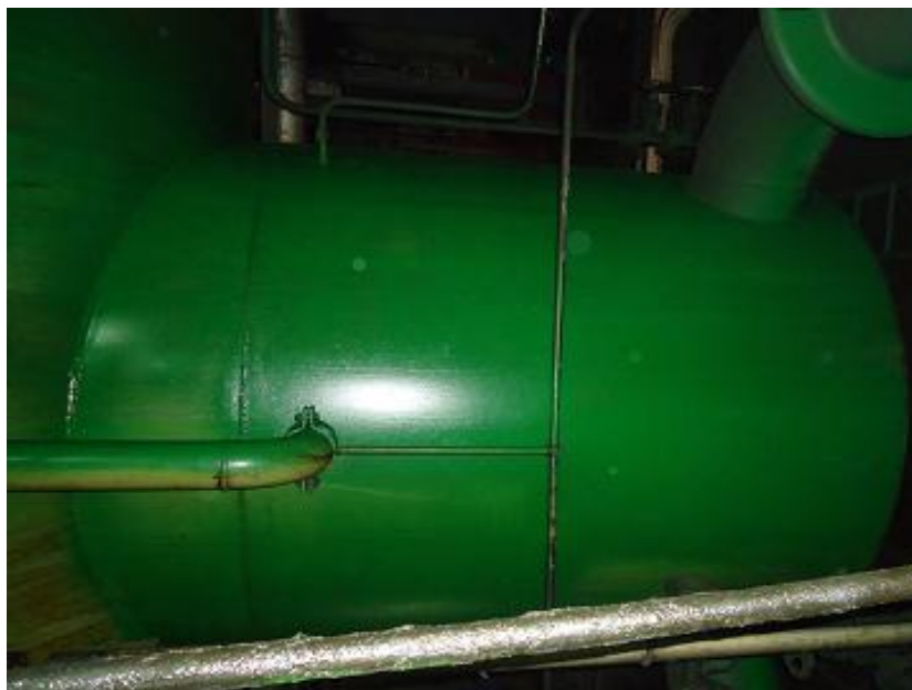
Figure 2.13: Hot well tank.
