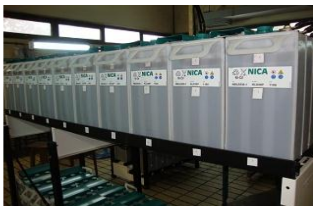
Figure 3.5: Batteries stacked in the battery backup room.
