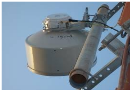
Fig 3.2: ODU with MW antenna in a BTS tower.
