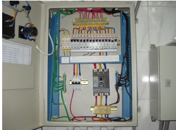
Fig 6.2: Main Distribution Board in BTS room.
