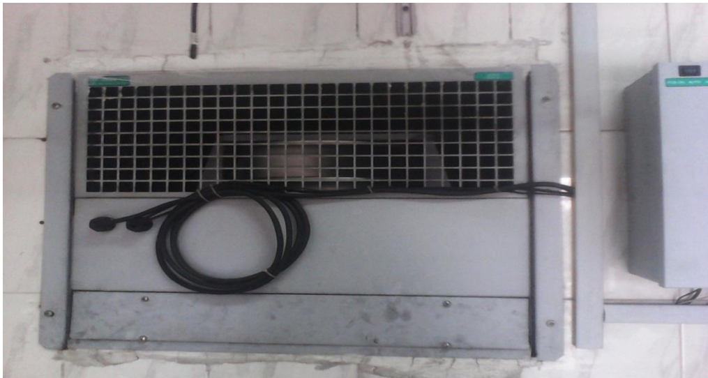
Fig 3.4: DVS at BTS room
