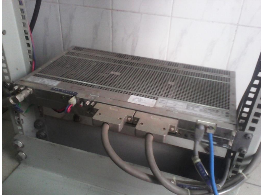
Fig 3.1: IDU in a BTS room.
