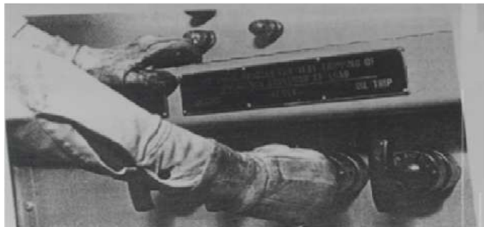
Figure 5. 12: Operator activating manual trip.
