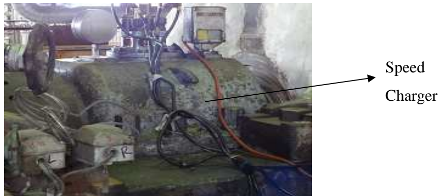
Figure 5.5: Speed Charger at unit 1.
