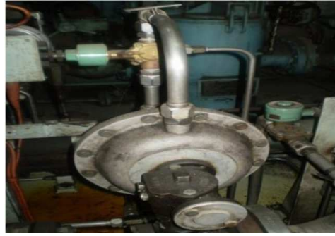
Figure 2.5: Pneumatic valve at unit 5.
