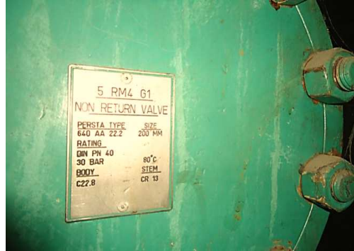
Figure 2.3: Non- Return valve at unit 5.
