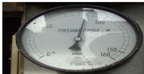
Figure 5. 9: Pressure gauge at unit 1.
