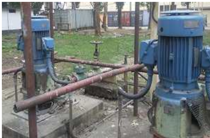
Figure 4.13: Drainage pumps of waste water basin at unit 3.
