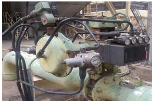
Figure 2.6: Temperature controlled valve of waste water basin at unit 3.
