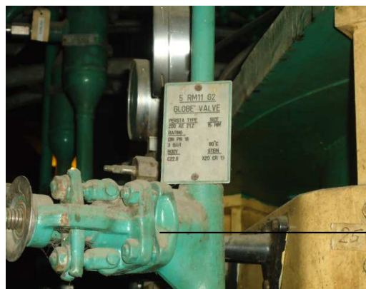
Figure 2.4: Globe valve at unit 5.
