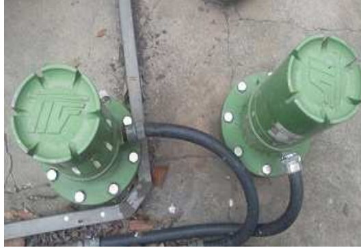
Figure 4.14: Water level sensor of waste water basin at APSCL.
