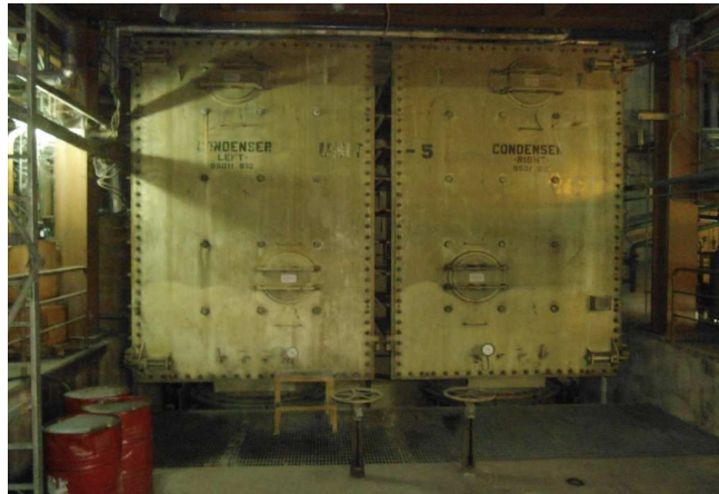
Figure 3.6: A Condenser at APSCL.
