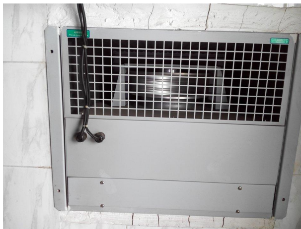
Fig07: DVS at BTS room
