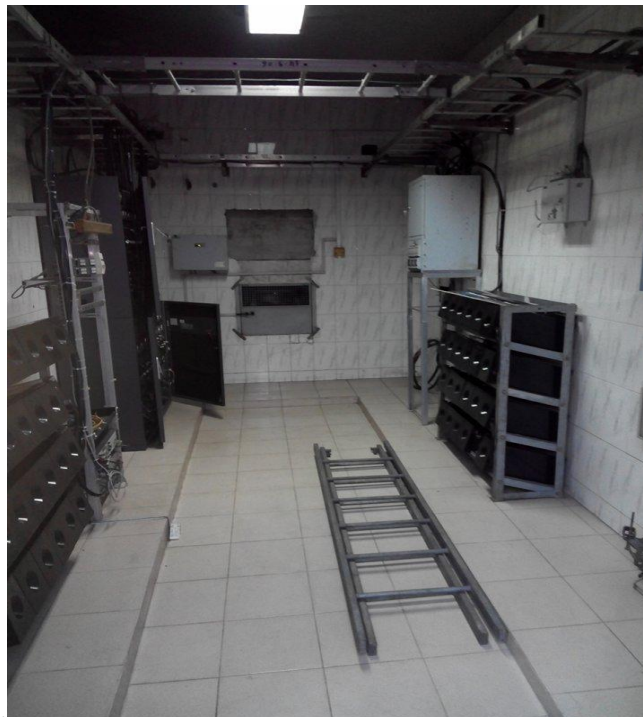
Fig23: Indoor BTS room
