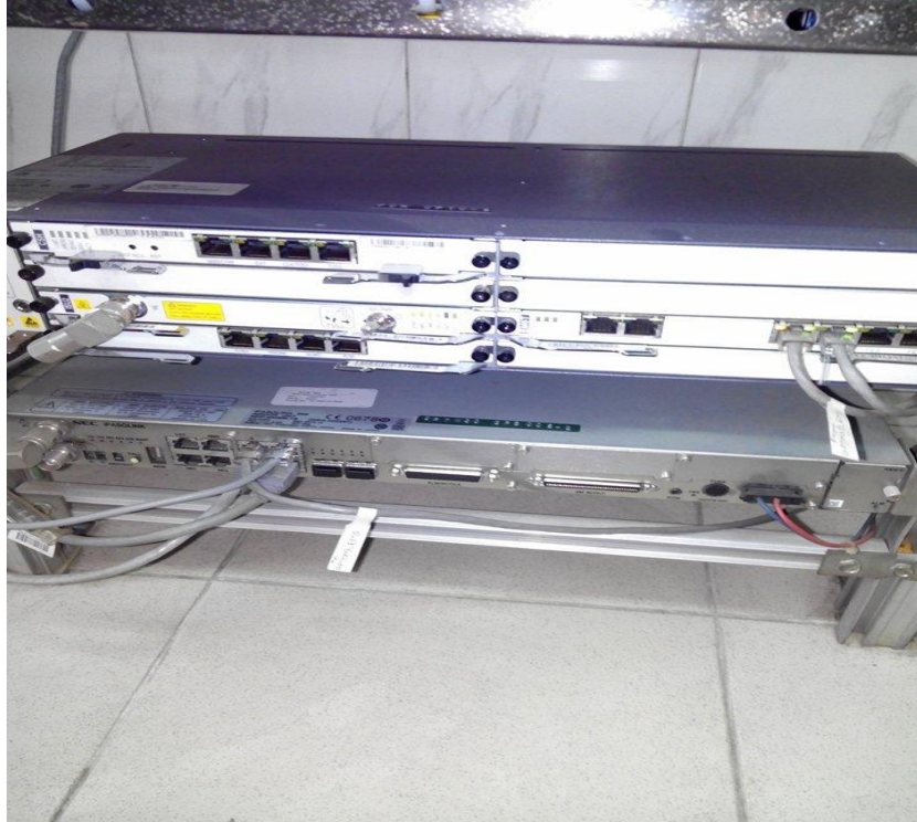
Fig01: IDU in a BTS room.
