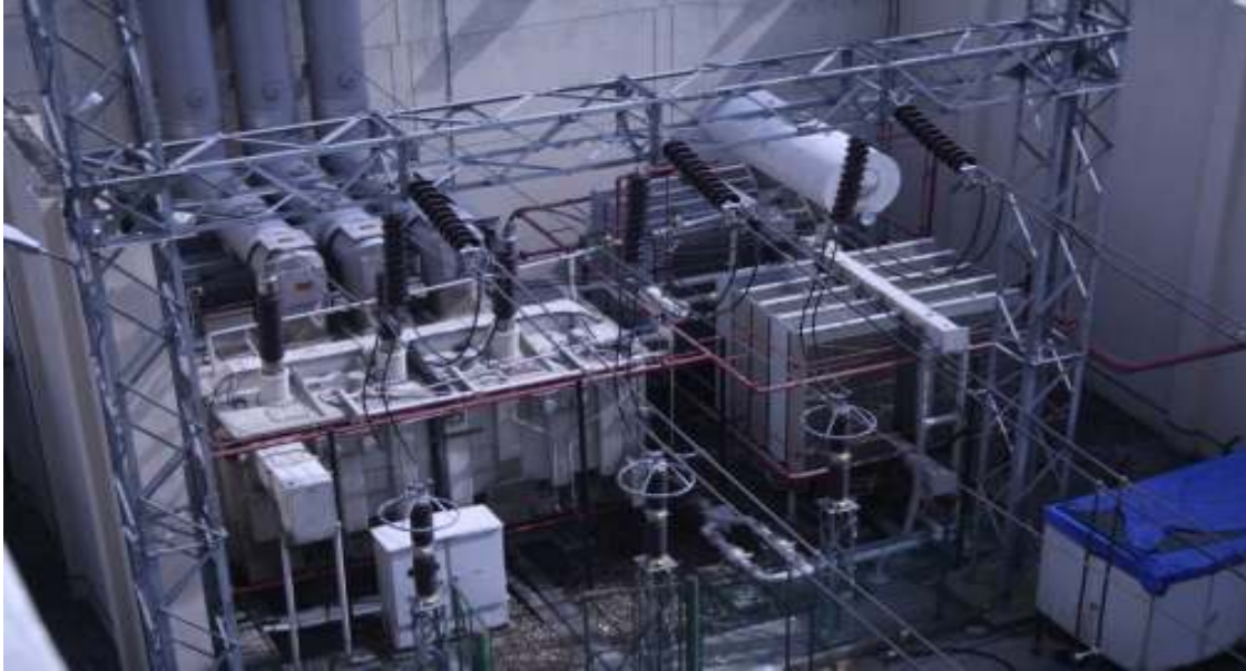
Figure 4.2: 11 KV/132 KV transformer used in Siddhirganj Peaking Power Plant [2].
