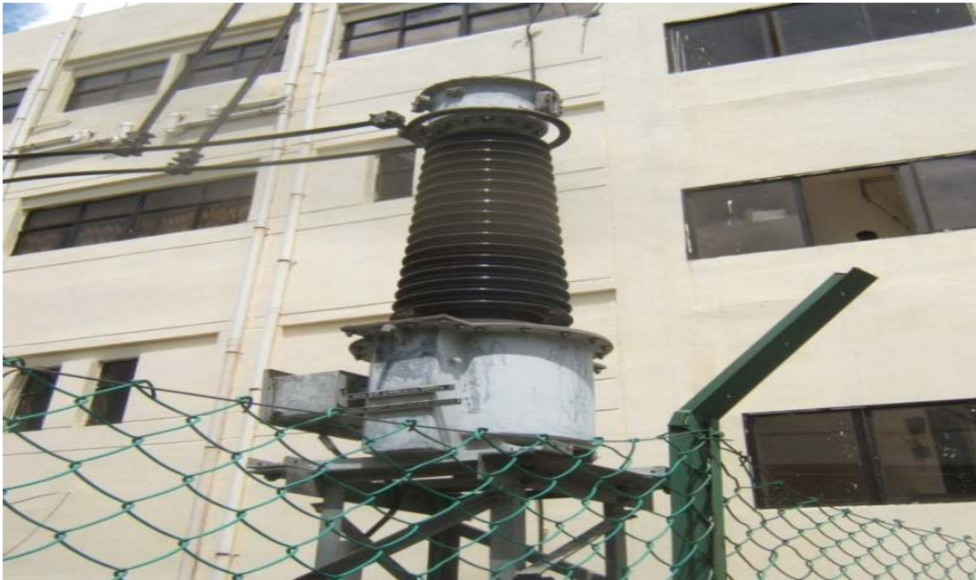
Figure 3.5: Picture of potential transformer used in Siddhirganj Power Plant [2].
