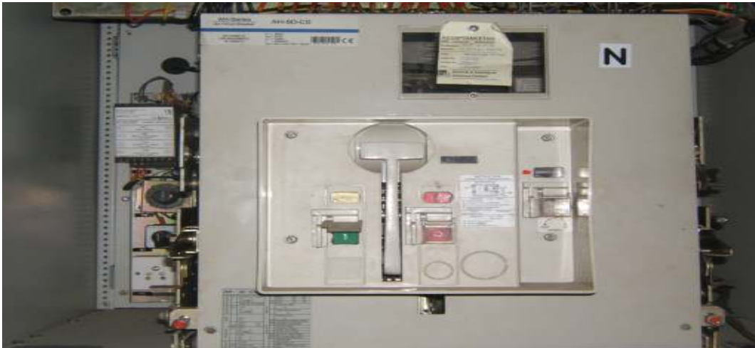
Figure 3.7: ACB used in Siddhirganj Peaking Power Plant [2].
