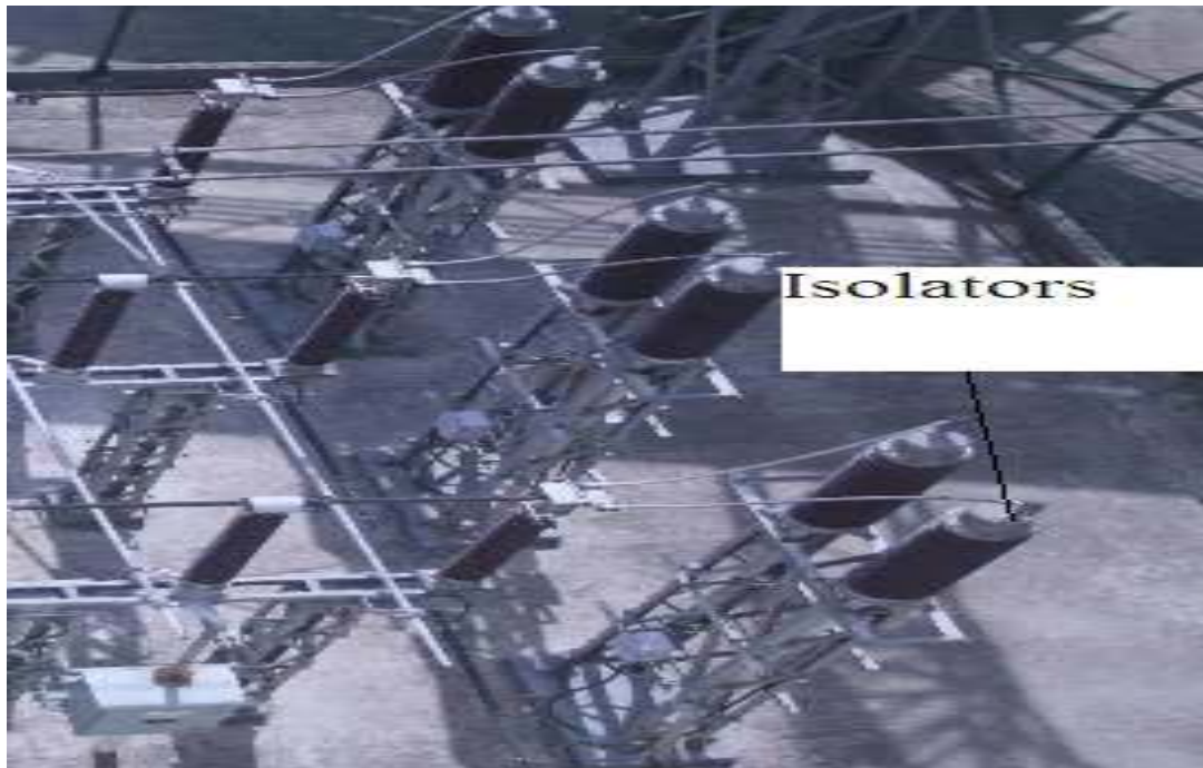
Figure 3.3: Picture of isolator in high voltage switch yard [2].
