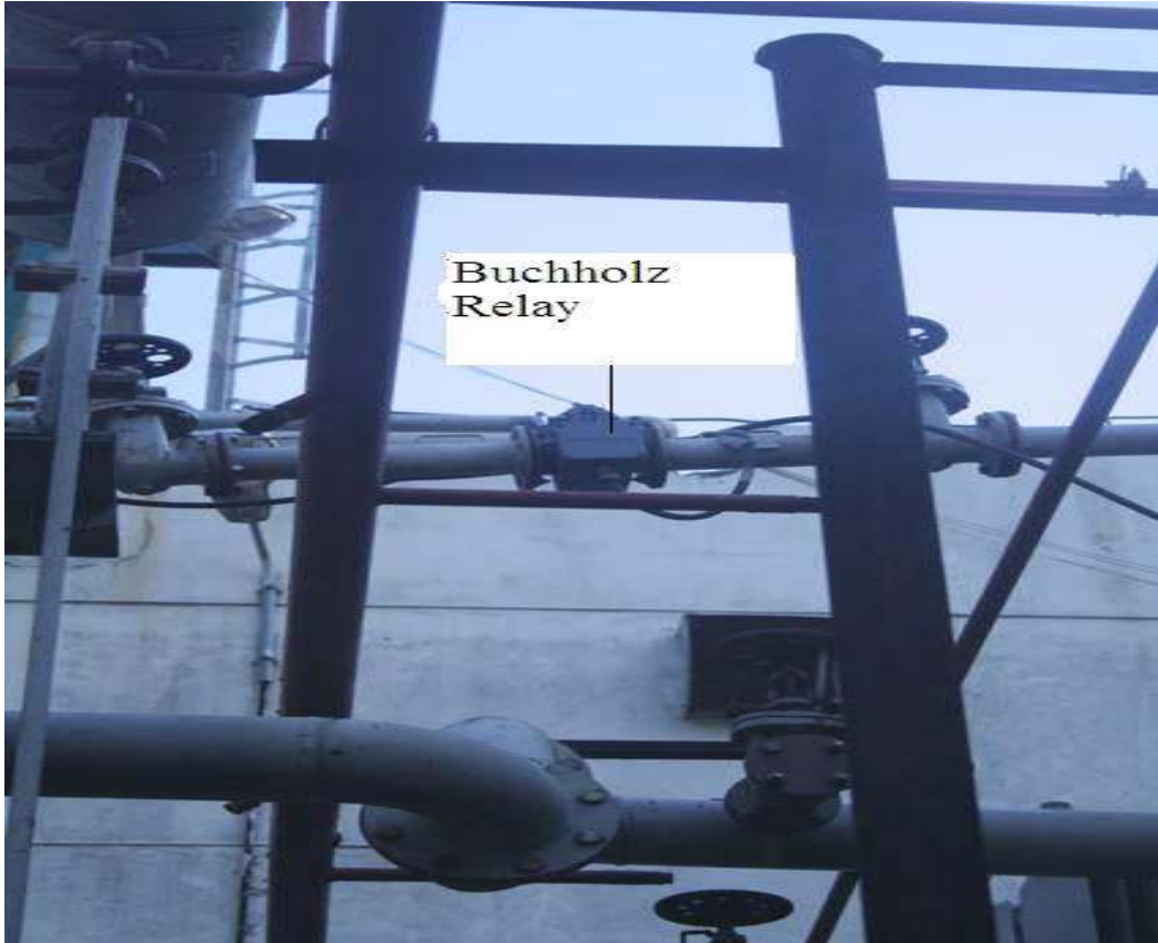
Figure 3.1: Buchholz relay in 132 KV transformers [2].
