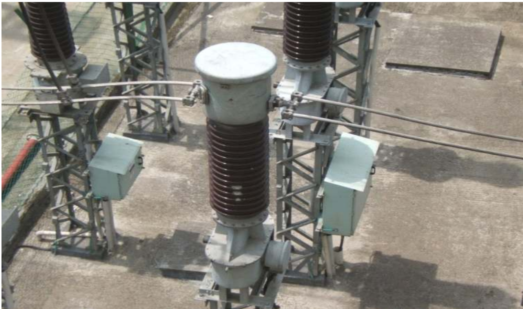
Figure 3.4: Picture of current transformer used in Siddhirganj Power Plant [2]. In figure (3.4) we can see three phase current transformer in high voltage switchyard.
