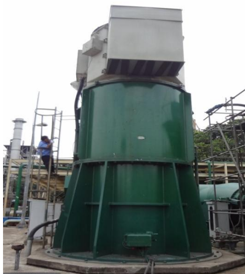
Figure 3.6: CW pump (unit-3) [5].
