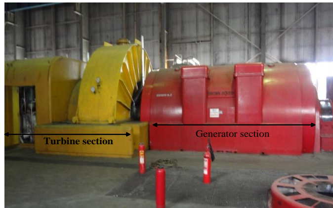
Figure 4.2: Turbine and generator of a boiler [5].
