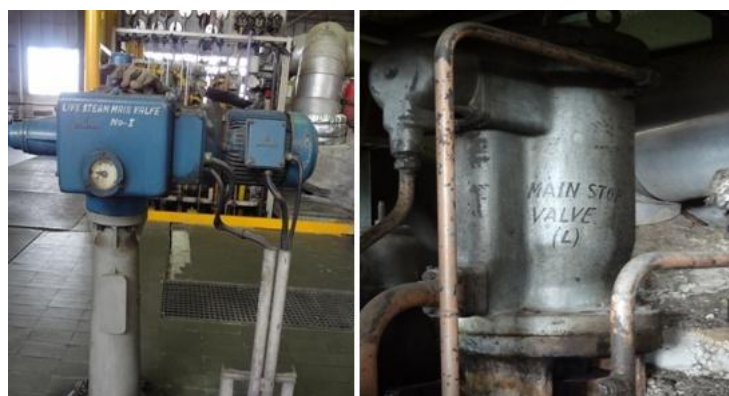
Figure 4.3: Live steam valve and main stop valve [5].
