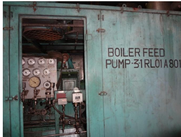
Figure 3.5: Boiler feed pump [5].
