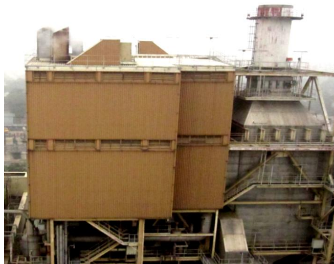
Figure 3.1: Boiler of APSCL [5].
