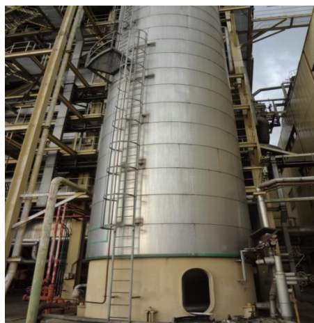
Figure 3.9: Storage tank of a boiler [5].
