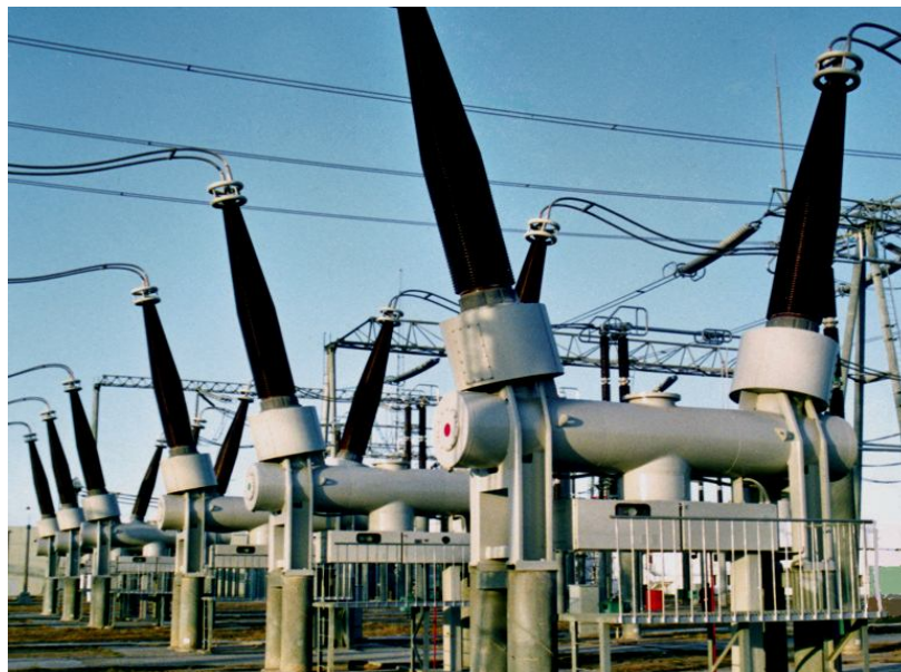
Figure 5.6: SF 6 circuit breaker with normal rated current is 1250 A
