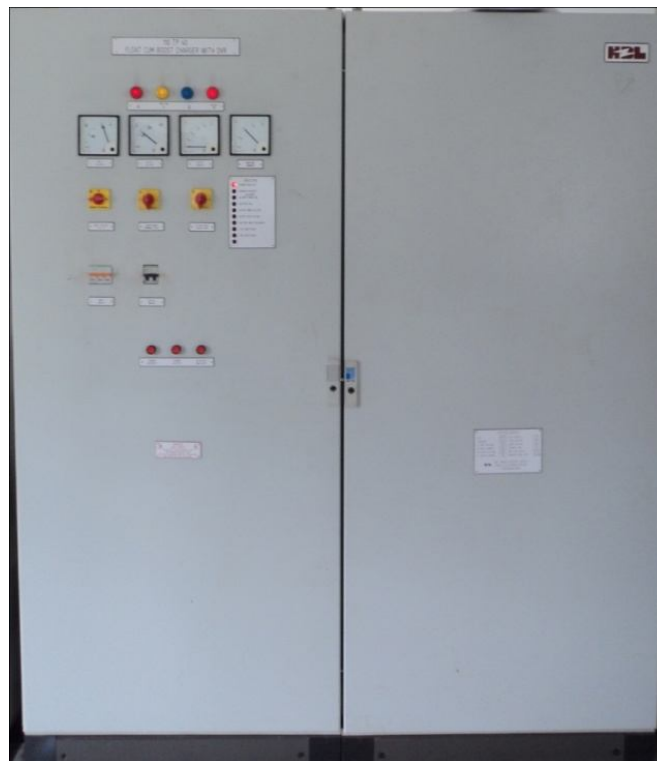
Figure 8.11: 110 TP 40 float CUM boost charger with DVR
