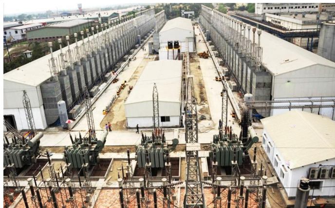
Figure 1.1: Desh Energy Limited at Shiddhirganj
