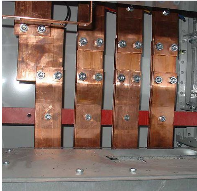
Figure 5.5: Bus bar connection of 132 KV line
