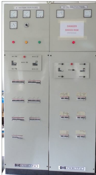
Figure 8.8: AC and DC distribution panel
