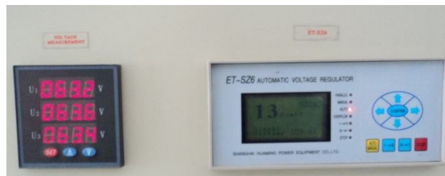
Figure 8.7: Automatic voltage regulator panel
