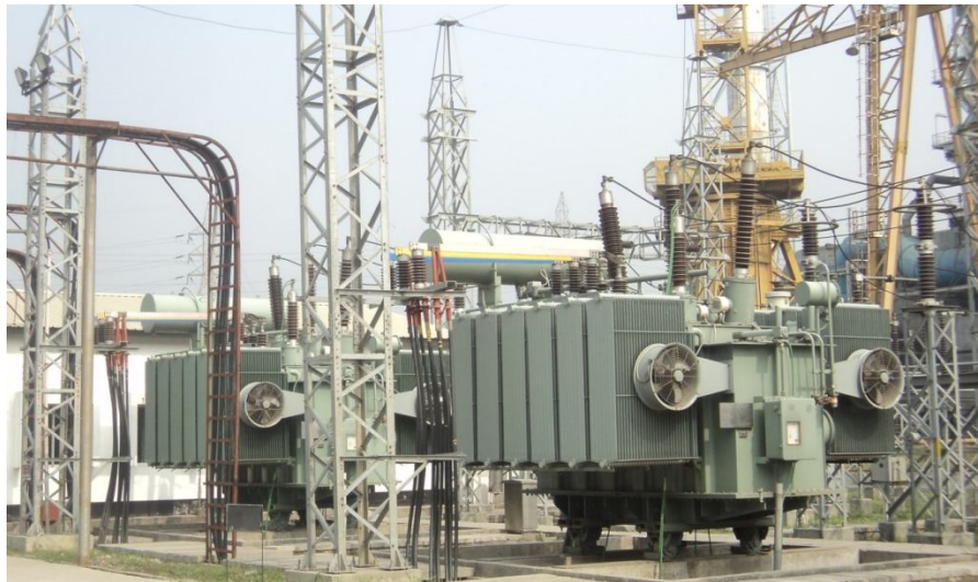
Figure 5.1: Site view of 11/132 KV DEL substation
