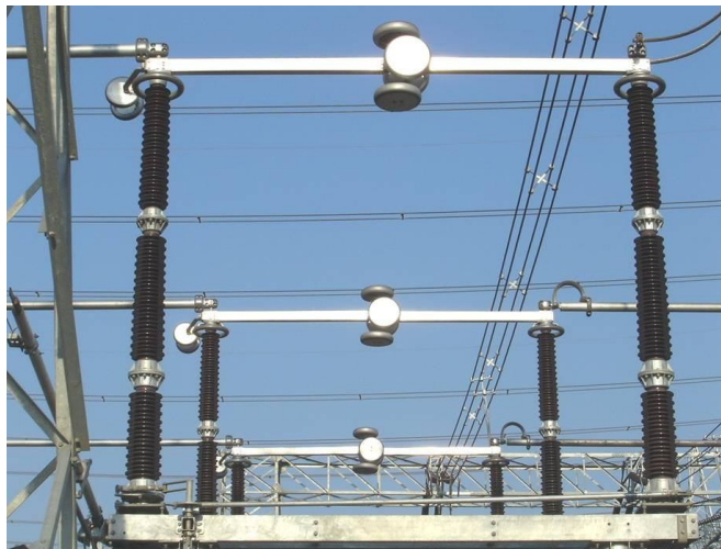
Figure 5.8: Electrical motor mechanism isolators
