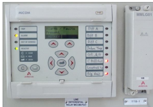
Figure 8.9: Line differential relay panel
