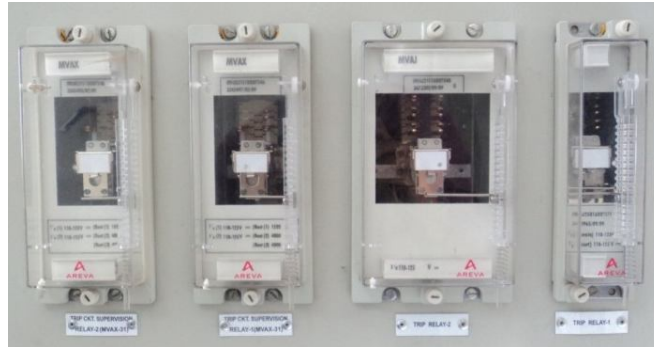
Figure 8.10: 132 KV outgoing feeder relay panel
