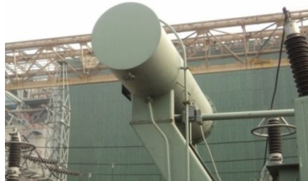
Figure 9.1: Oil tank of a transformer
