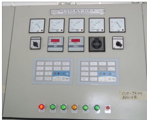
Figure 8.12: 11 KV/132 KV GT control panel – upper part
