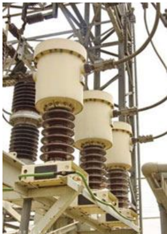
Figure 5.3: 100:5 A Current transformer
