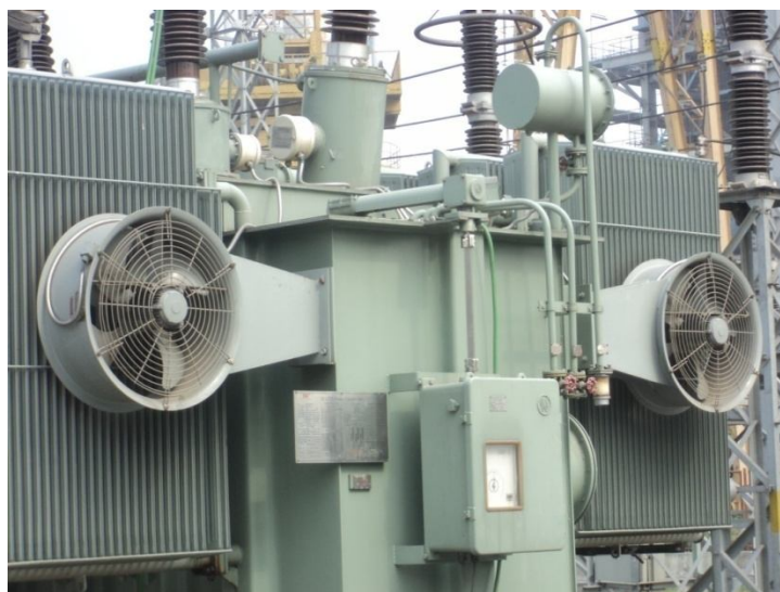
Figure 5.2: Three phase, 35000 KVA, 11KV/132KV, 50 Hz power transformer.
