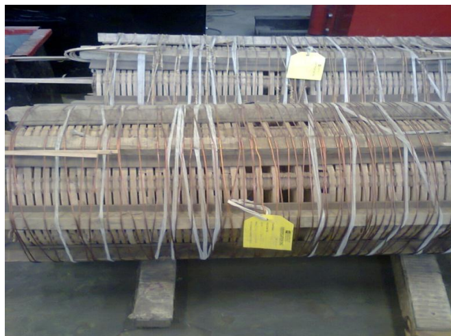
Figure 2: Transformer LT coil
