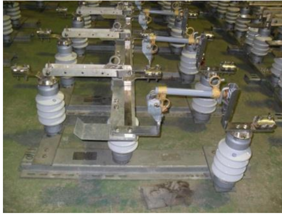
Figure 30 : Auto Circuit Reclosure Switches
