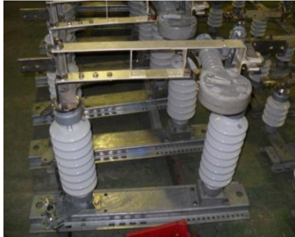
Figure 28 : Air Break Switch with Load Interrupter
