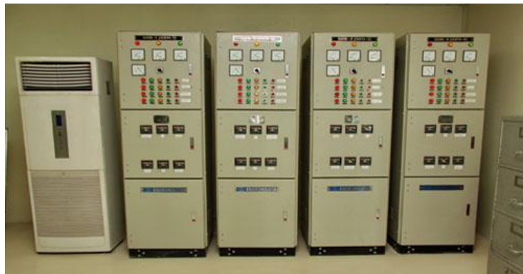
Figure 11: LT switchgear panel
