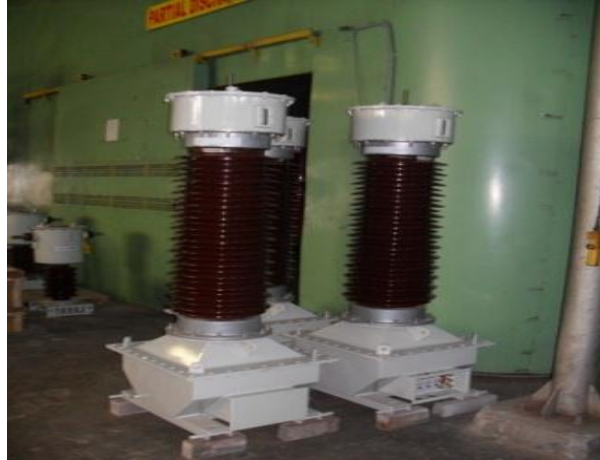
Figure 23 : Outdoor Potential Transformer
