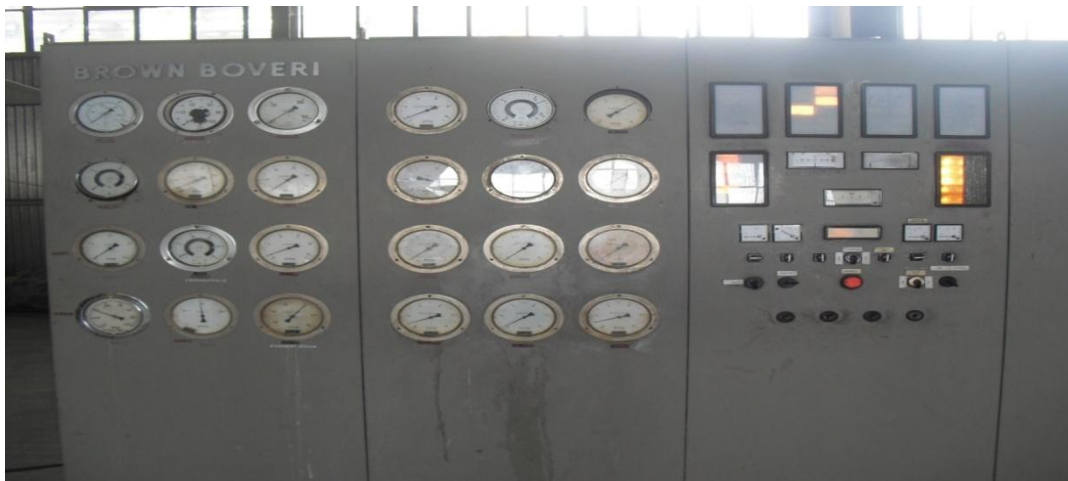
Figure 3.1: Operation unit of control unit 1 and 2.
