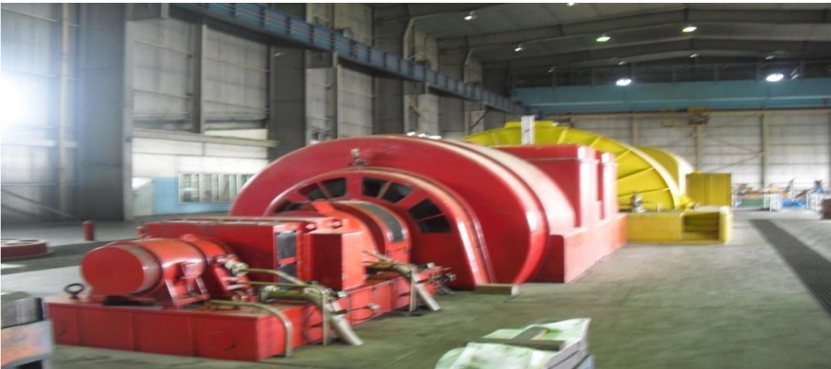
Figure 2.1: The whole generator of control room 1 (unit 1 and 2).
