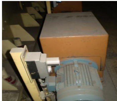
Figure 2.4: Jacking oil pump.
