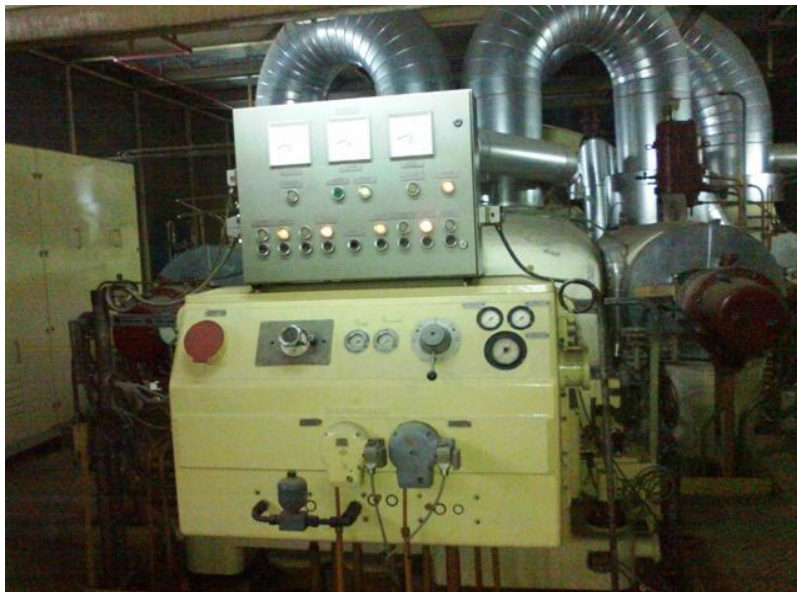
Figure 5.9: Low pressure system turbine in unit 3.
