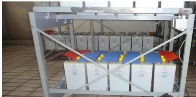
Figure 4.6: Parallel connected battery.
