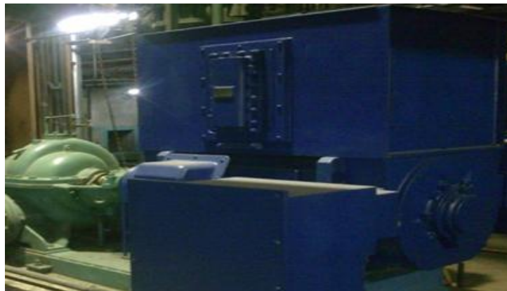
Figure 4.9: Water cooling pump used for water cooling at APSCL.
