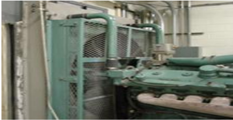
Figure 4.10: Air cooling system in APSCL using external fan.
