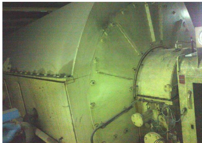
Figure 5.8: High pressure system turbine in unit 3.
