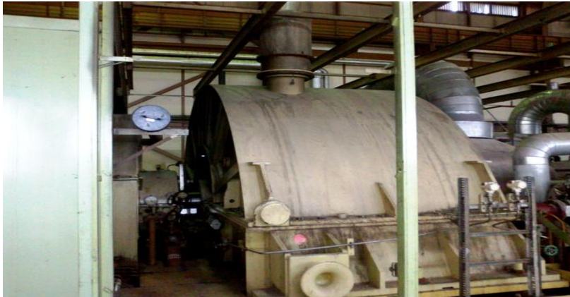
Figure 5.7: Turbine of unit 1.
