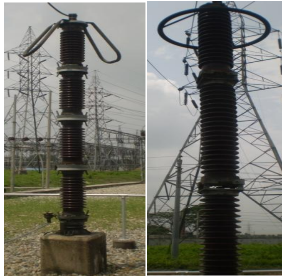
Figure 5.12: Picture of Lightning arrester.
