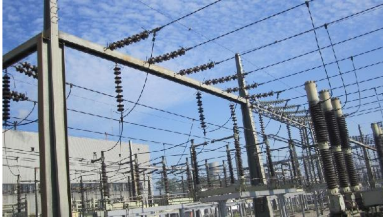
Figure 5.28: 230KV Double circuit bus bar.
