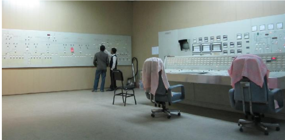
Figure 4.21: Control room at APSCL.
