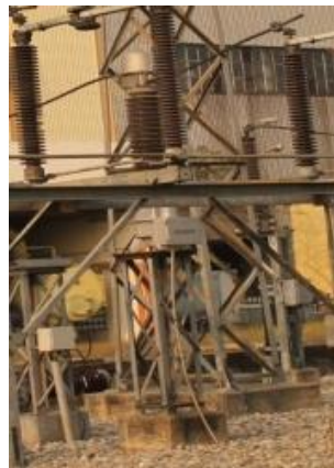
Figure 5.13: Earthing switch used in 132KV line.
