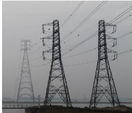
Figure 5.19: High voltage double circuit transition line.
