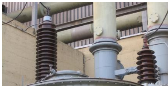
Figure 5.14: Rod gap type lightning arrester of APSCL.
