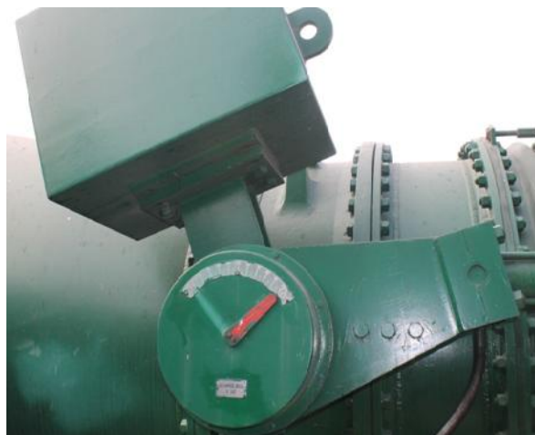
Figure 3.4: Water flow control valve.
