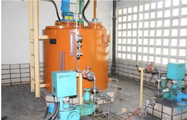
Figure 2.15: Water treatment plant in APSCL.
