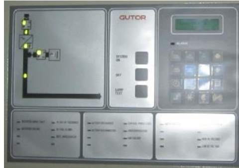
Figure 5.23: Rectifier used for battery charging purpose.
