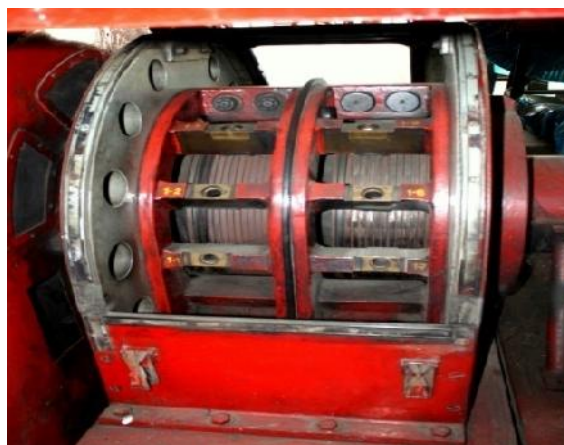
Figure 2.2: DC Exciter used in 150 MW generator of unit 3.
