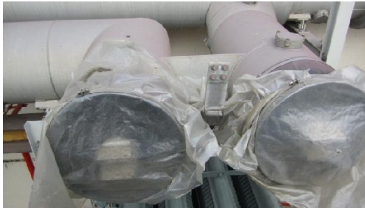
Figure 5.24: Conductors which contains 4000A current.
