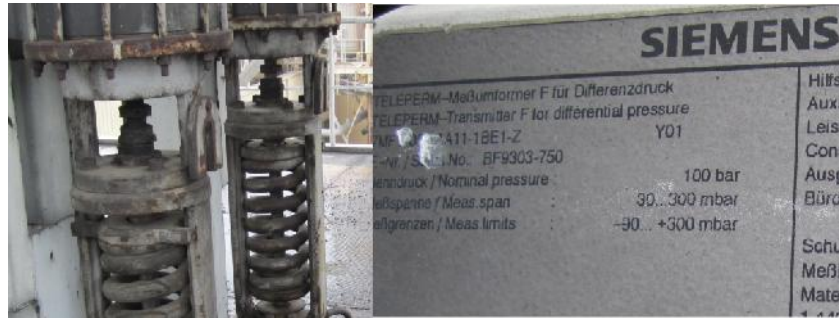
Figure 4.12: Steam pressure safety valve of boiler.
