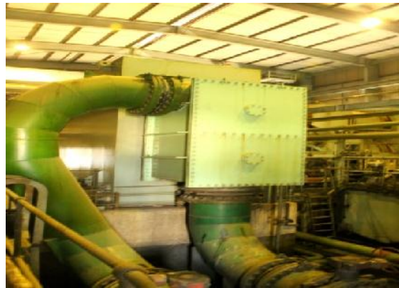
Figure 2.18: Condenser in steam turbine of 34 MW & 13.8 KV in CCPP.
