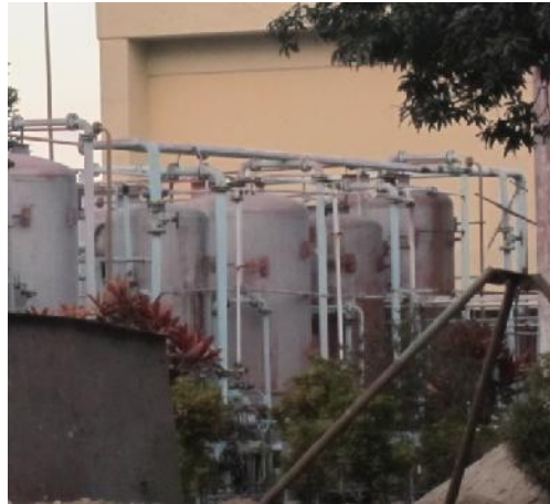
Figure 4.7: Hydrogen supply station.
