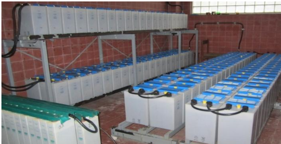
Figure 5.22: Dc battery room of APSCL substation.
