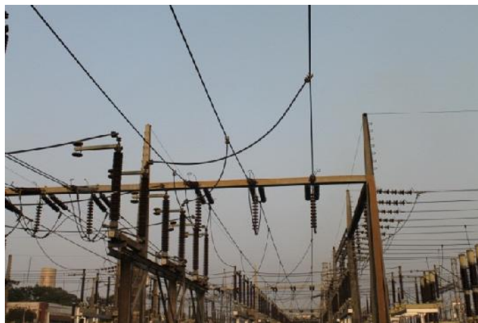
Figure 5.16: 132KV double circuit bus bar.
