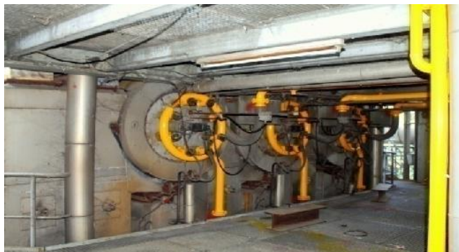
Figure 2.7: Burner used in 150 MW & 15.75 KV of APSCL.
