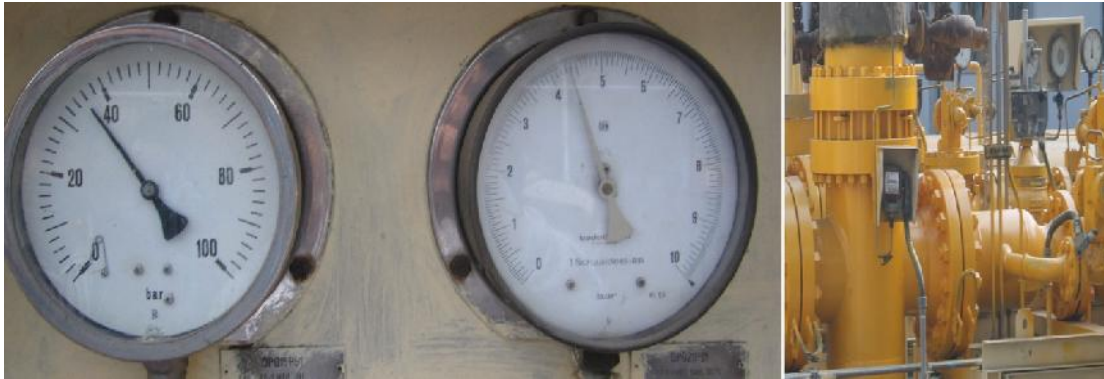
Figure 3.1: Gas pressure reducing valve.
