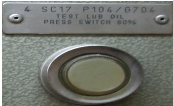
Figure 4.9: Lube oil pressure control switch.
