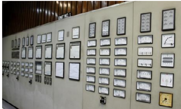
Figure 2.20: Analog monitoring parts of 64 MW & 11 KV unit 1.
