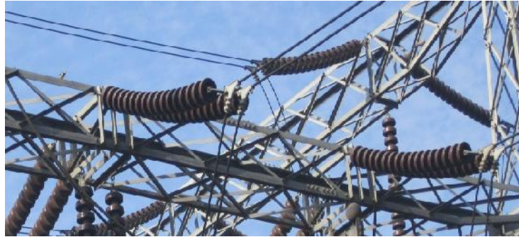
Figure 5.18: Suspension type insulator observed from APSCL substation.
