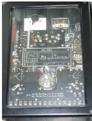
Figure 4.3: Under frequency relay.
