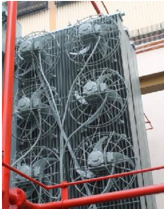
Figure 5.3: Radiator of a power transformer.
