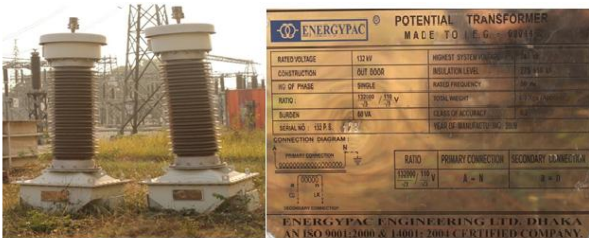
Figure 5.6: Potential transformer with nameplate of the APSCL substation.
