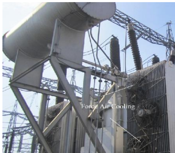
Figure 4.17: Forced air cooling system of transformer.
