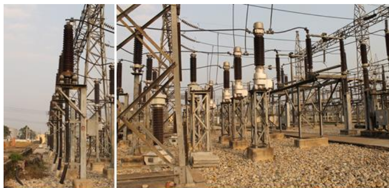
Figure 5.27: Typical 230KV feeder for unit three.
