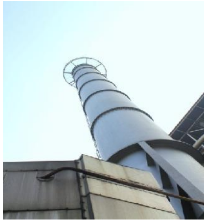
Figure 2.14: Chimney in 64 MW & 11 KV units 1.
