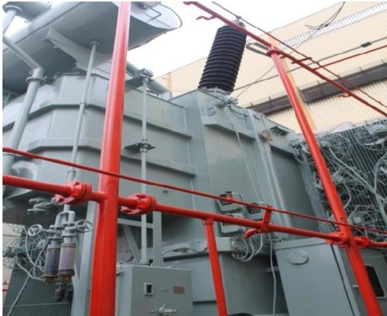
Figure 5.2: Tap changing power transformer.
