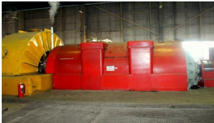
Figure 2.1: 150 MW AC generator of unit 3 .
