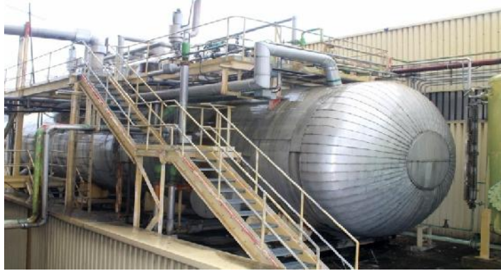
Figure 2.16: Deaerator in 150 MW & 15.75 KV unit 3 at APSCL.
