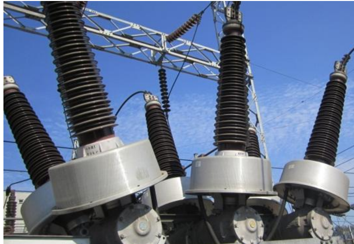
Figure 5.12: SF6 circuit breaker.
