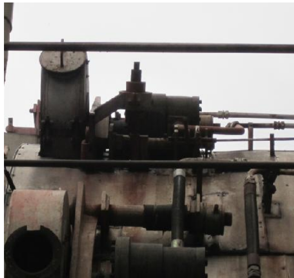
Figure 4.13: Flue gas damper of boiler.
