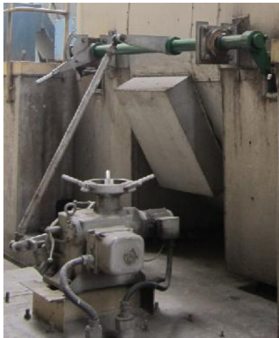
Figure 3.3: FD fan air flow control valve.
