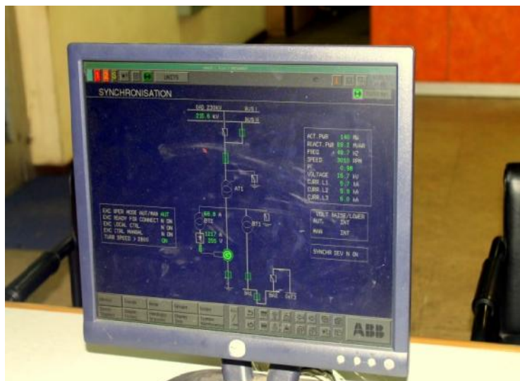
Figure 2.23: Software based control system in 64 MW & 11 KV unit 5.
