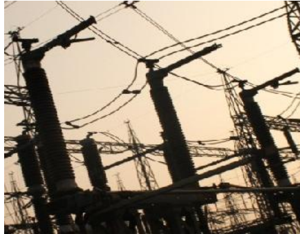
Figure 5.10: Horizontal center break isolator from APSCL.
