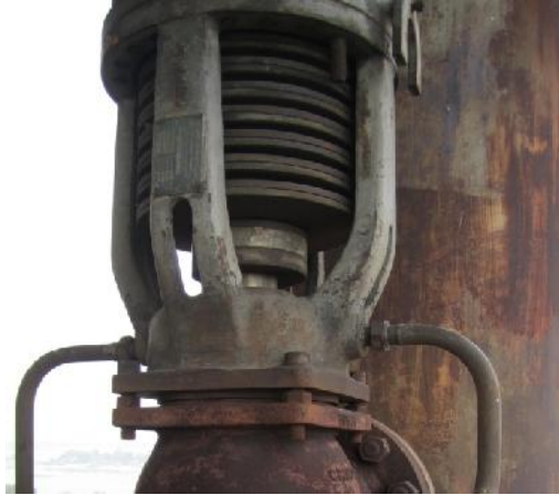
Figure 3.5: Super heater safety valve.
