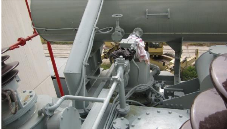
Figure 5.26: Output bushing of the single phase unit transformer.
