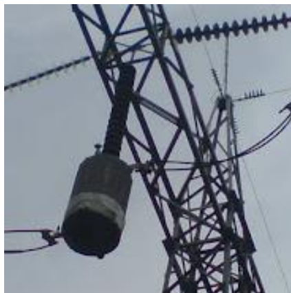
Figure 5.21: Wave trap used on APSCL substation.
