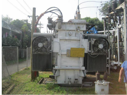
Figure 2.7: Transformer with cooling system
