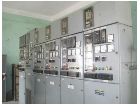
Figure 4.6:33/11KV Circuit Breaker
