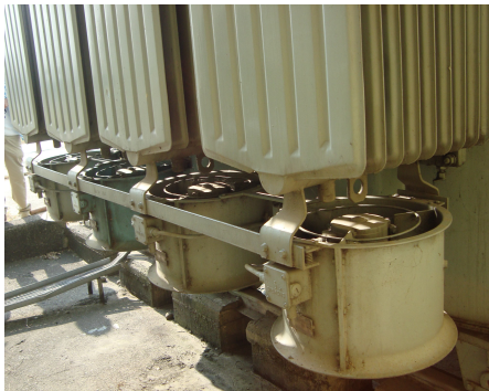
Figure 5.13: Transformer cooling fans
