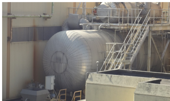
Figure 2.11: Feed Water tank in APSCS
