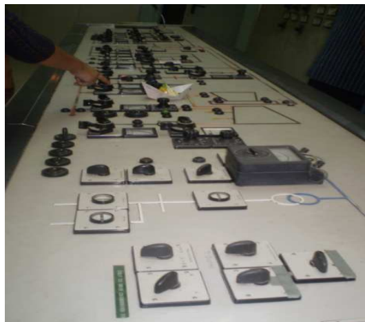
Figure 4.1: Operation unit of control unit 1 & 2
