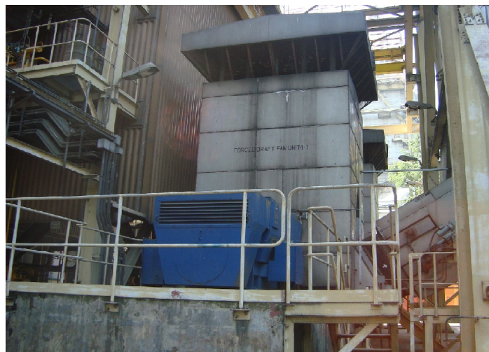
Figure 2.13: FD fan in APSCL
