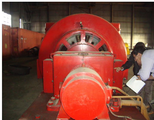
Figure 2.1: Steam Turbine Generator in APSCL
