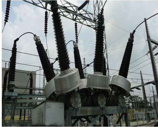
Figure 5.9: SF6 Circuit Breaker in APSCCL
