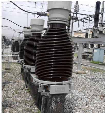
Figure 5.4: Potential Transformer in APSCl
