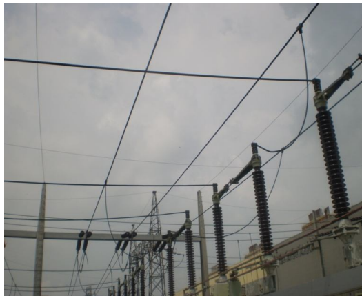
Figure 5.7: An Isolator in APSCL
