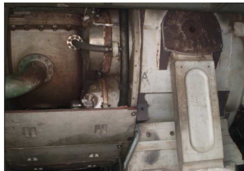
Figure 2.18: Combustion Chamber of Gas Turbine Plant of APSCL
