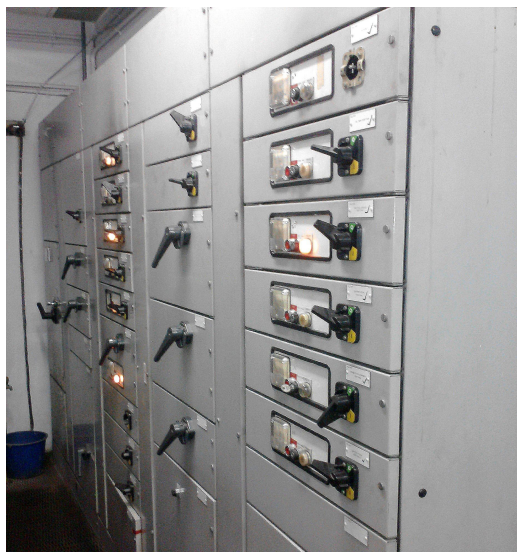
Figure 4.8: Switchgear unit of combine cycle plant.
