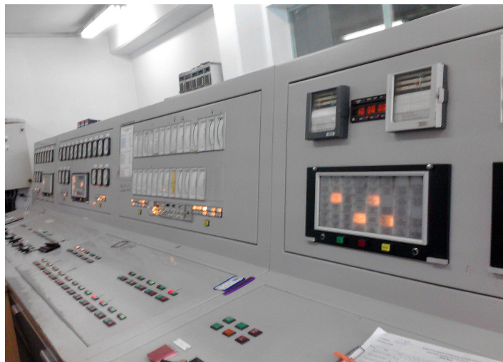
Figure 4.7: Control unit of combined cycle plant.
