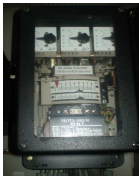
Figure 3.1: Overcurrent relay in APSCL
