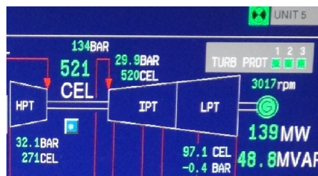
Figure 2.7: Turbine assembly in Unit-5 zoomed in from the Water & Steam Cycle
