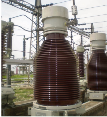
Figure 5.3: Current Transformer in APSCl
