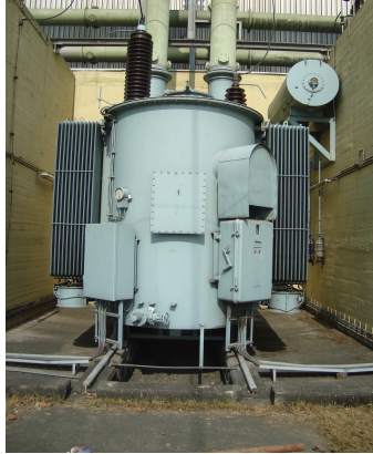
Figure 5.1: Power Transformer in APSCL
