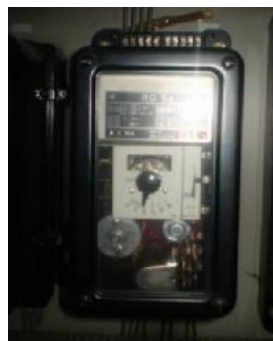
Figure 3.3: Stator Earth Fault relay
