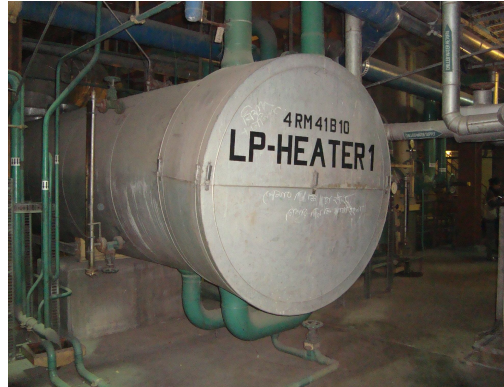
Figure 02.10: LP Heater-1 in APSCS steam power plant
