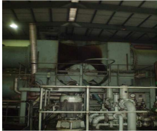
Figure 2.19: Gas turbine of APSCL
