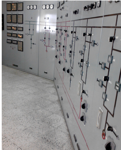
Figure 4.9: Control unit of sub-station
