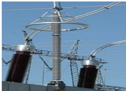
Figure 5.11: Lightning Arrester in APSCL
