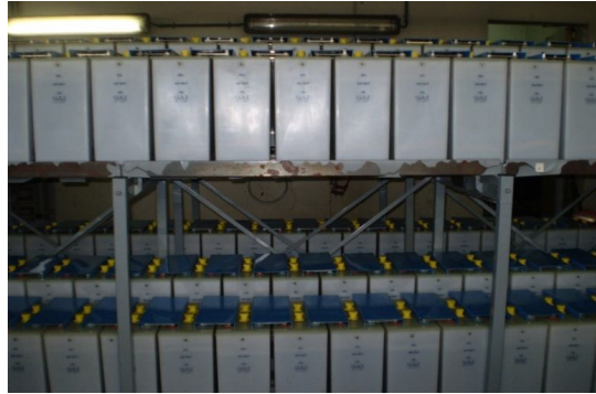
Figure 5.14: Battery Arrangement of back-up system in APSCL
