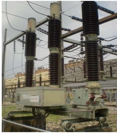
Figure 5.8: Oil Circuit Breaker in APSCL
