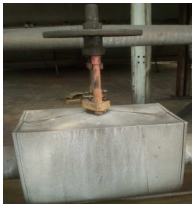
Figure 2.21: Manual valve used in combined cycle power plant of APSCL
