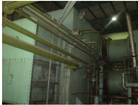
Figure 2.17: Centrifugal compressor used in APSCL
