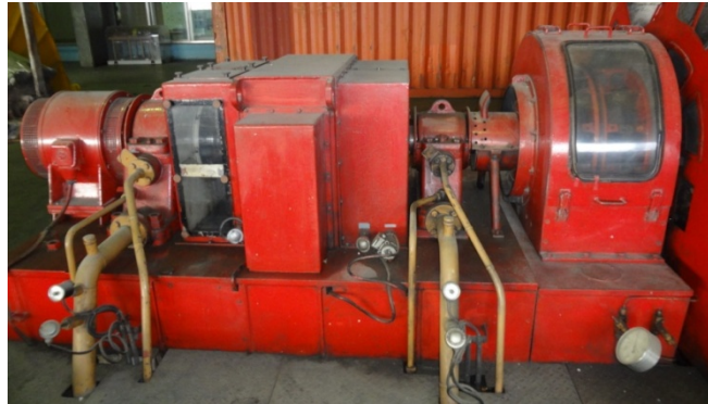
Figure 2:2: AC Generator of unit-2 APSCL.
