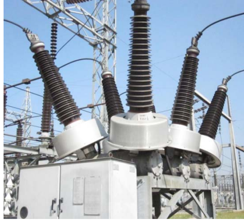
Figure 5:9: SF6 Circuit Breaker in APSCL
