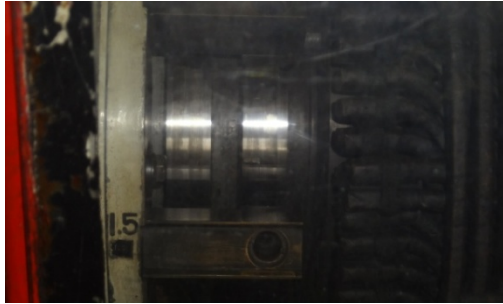
Figure 2:4: Generator slip rings of unit-5 in APSCL.
