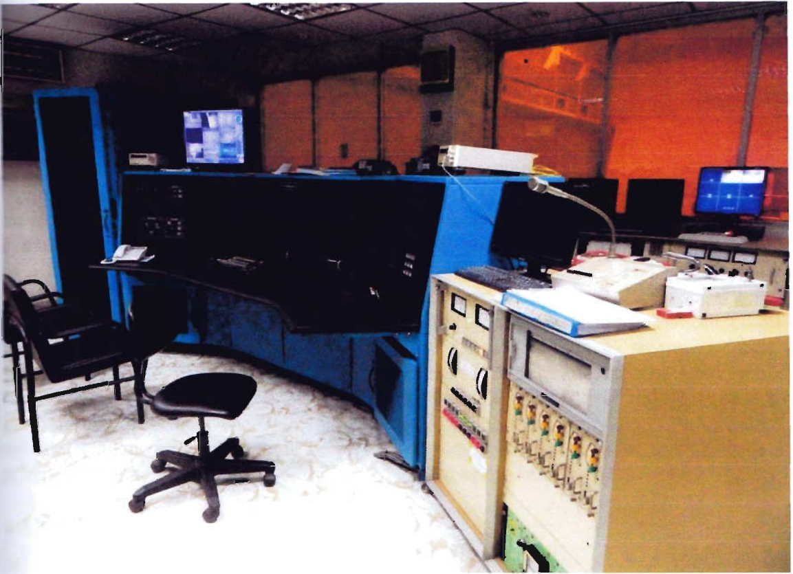
FIG 4.3: Control room of TRIGA MARK-II RESEARCH REACTOR.
